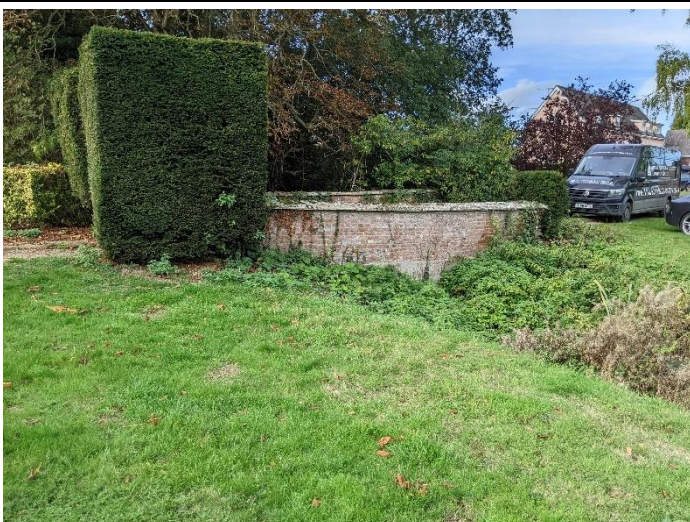
Photo 5 View of bridge to the north of Clopton Hall which will be demolished
