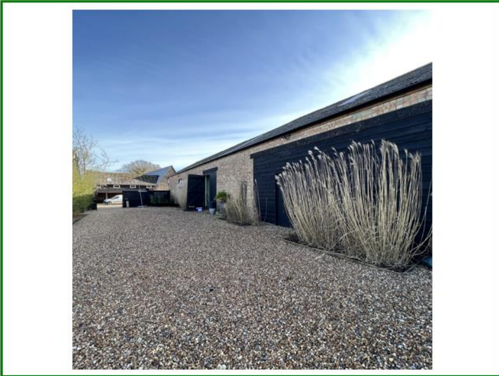
Photo No.4: Facing SE from outside the NW corner of the building on site showing the front (northern) face of the building
