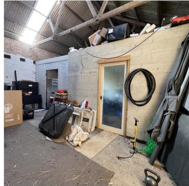
Photo No.12: Facing SW inside the barn unit showing interior rooms (location of gym equipment)
