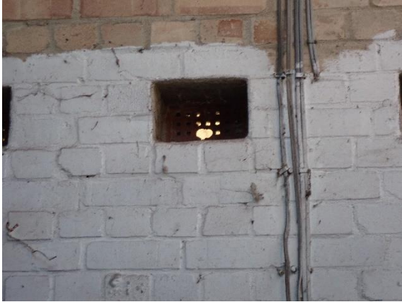
Damaged vent brick
