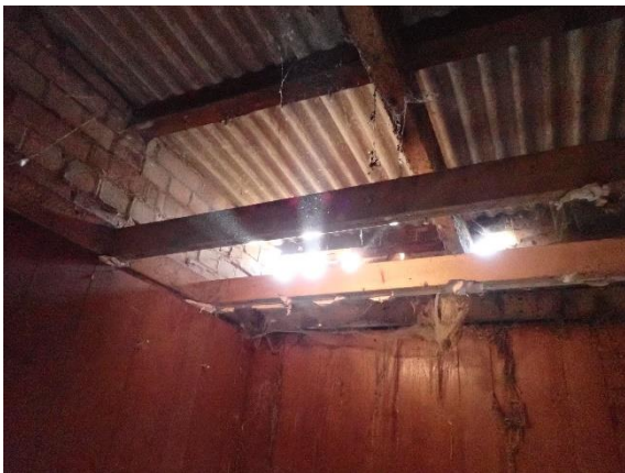
Damage at the top of walls providing ingress for bats
