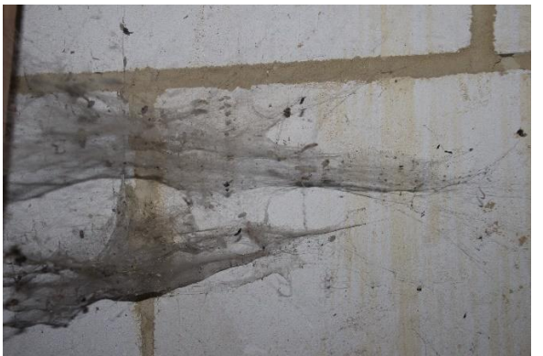
6. Bat droppings caught in web by chimney
