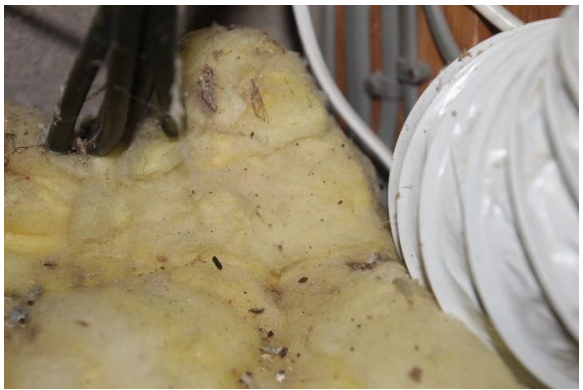
7. Bat dropping on insulation
