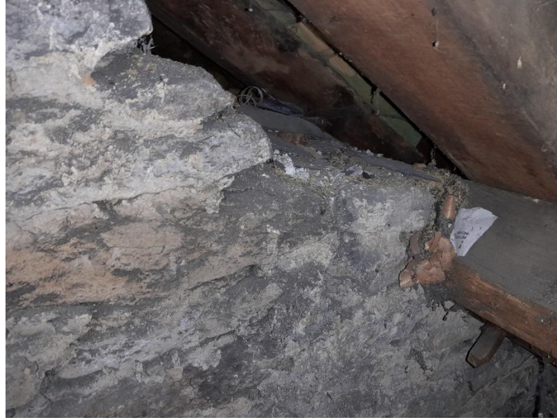
View to side of gap between wall head and underside of roof coverings.
