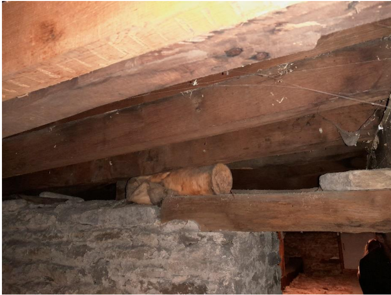
Gap to top of existing stone wall
