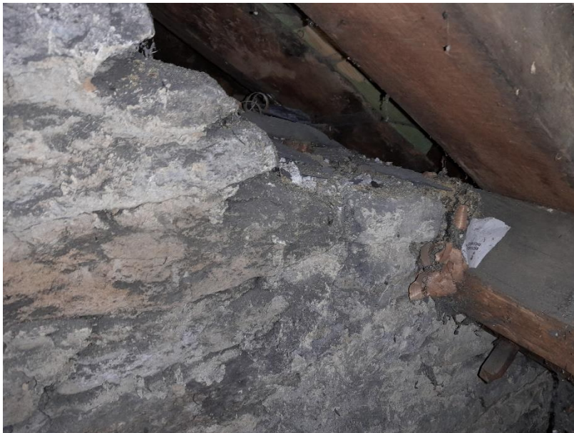
Gap to top of existing wall
