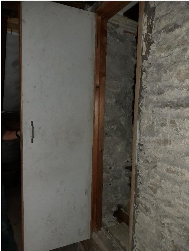
Modern door within roof void containing asbestos to be replaced.
