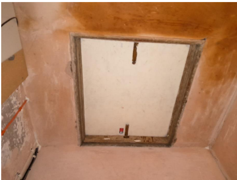
Modern hatch within roof void containing asbestos to be replaced
