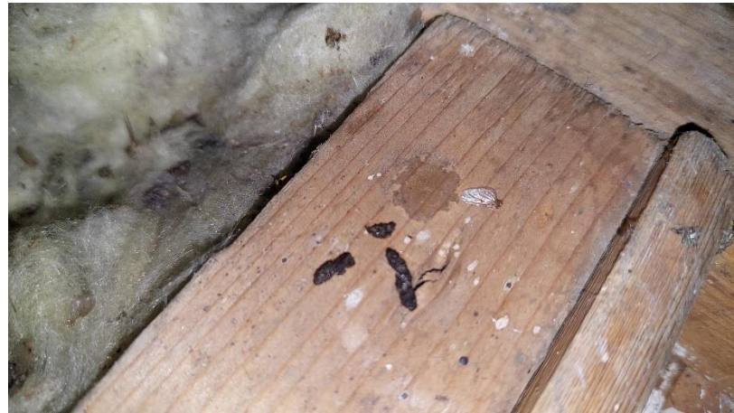
Photograph 19: Bat droppings on the floor recorded on the insulation of Loft 2.
