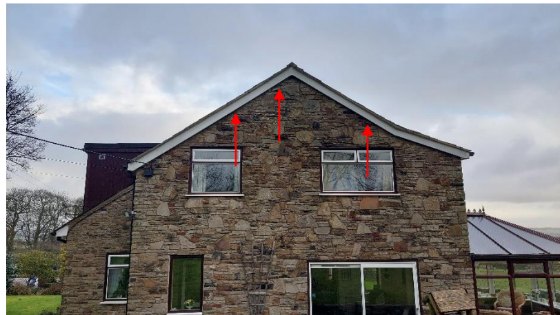
Photograph 23: Southern aspect of existing farmhouse. Red arrows indicate potential ingress/egress for bats.
