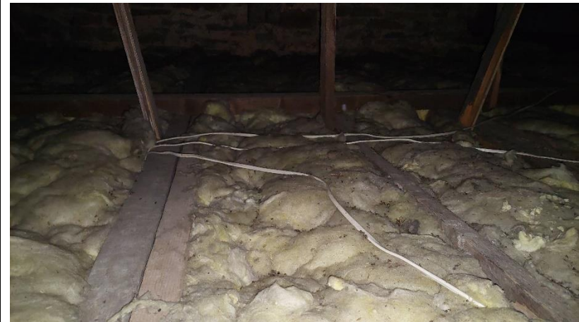
Photograph 16: Woollen loft insulation of Loft 2. Access was restricted but bat droppings were found on top of the insulation but these could not be more closely inspected than is seen in this photograph.
