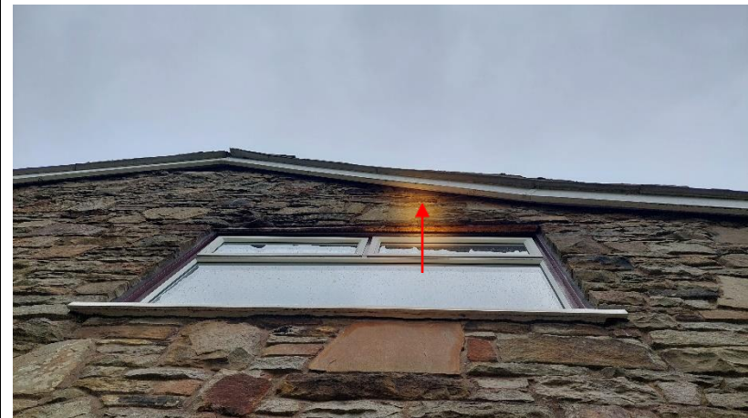
Photograph 24: Southern aspect of existing farmhouse (refer to Photograph 23 which includes the same larger double glazed, upstairs bedroom window). Red arrows indicate potential ingress/egress for bats.
