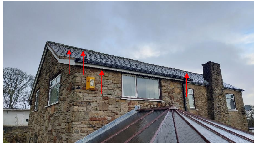
Photograph 25: Eastern aspect of the existing farmhouse. Red arrows indicate potential ingress/egress for bats.
