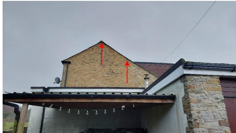
Photograph 27: Northern gable end of the existing farmhouse. Red arrows indicate potential ingress/egress for bats.
