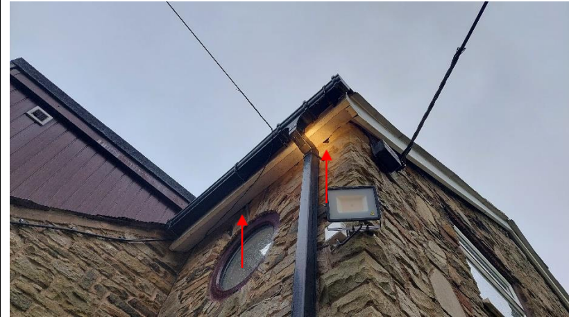
Photograph 22: Western aspect of existing farmhouse. Porthole window in this photograph is that which is in Photograph 21.
