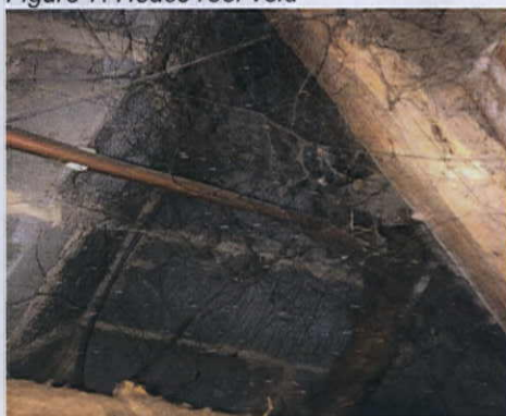
Figure 9: Dense cobwebbing around chimney
