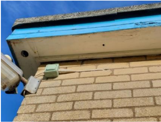
Plate 4.19: Missing vent cover
