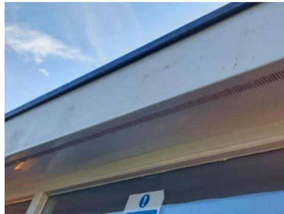
Plate 4.12: Gaps under roof edge
