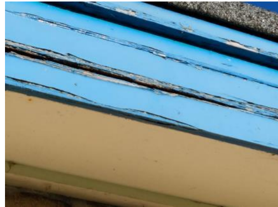
Plate 4.16: Gap in fascia board
