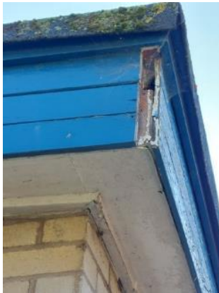
Plate 4.15: Damaged fascia boards
