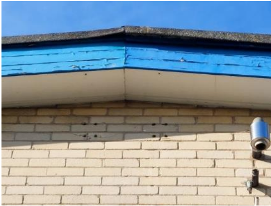
Plate 4.13: Gaps under roof edge
