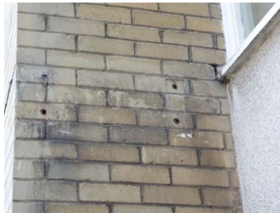
Plate 4.21: Holes in brickwork and gap around windowsill
