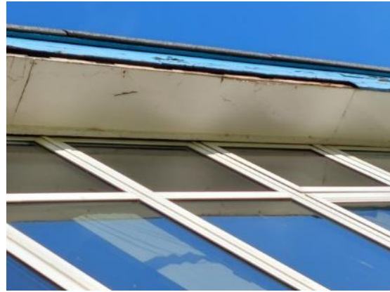
Plate 4.14: Damaged fascia boards
