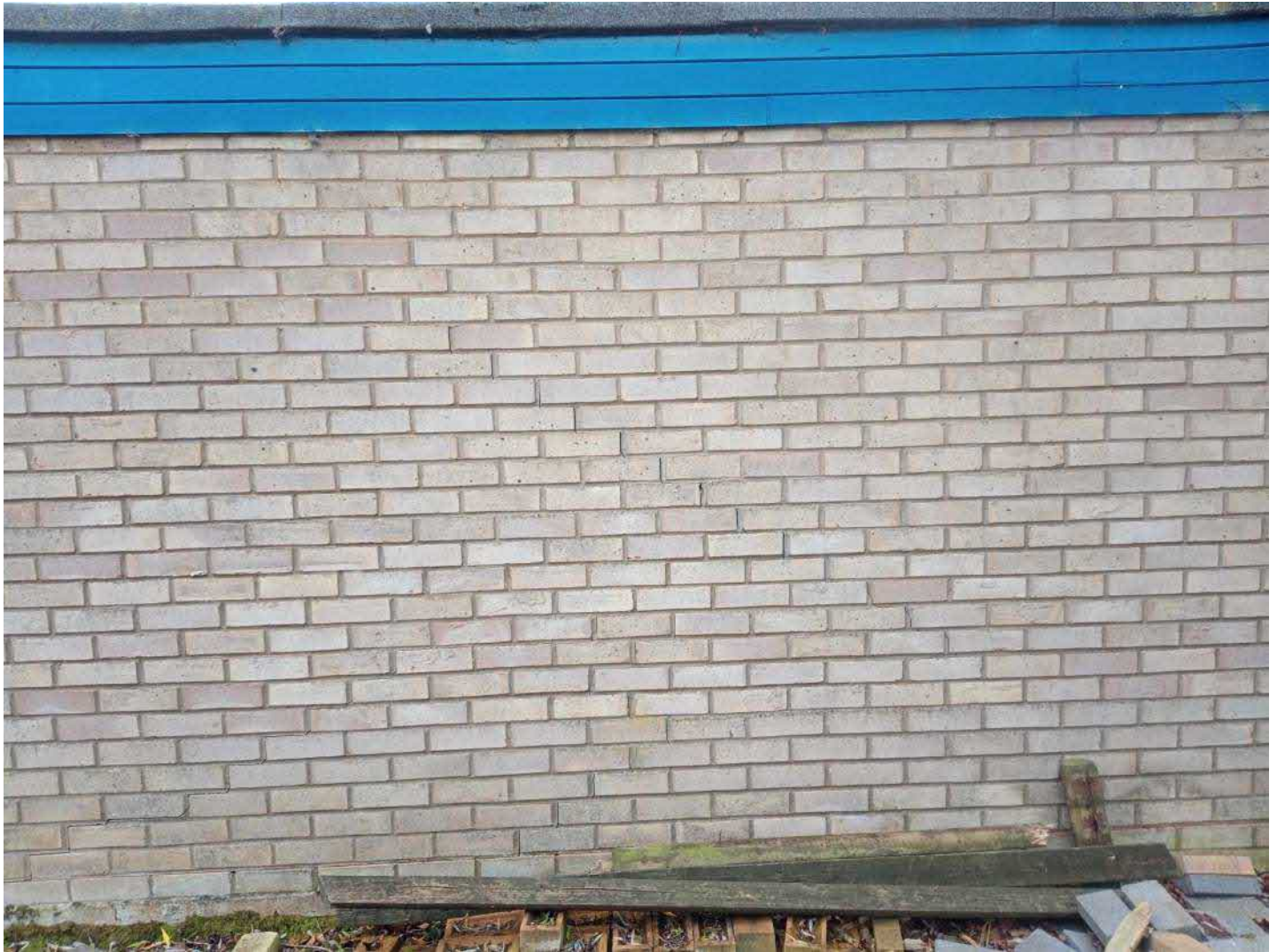
Location 06 facing South - Cracking on northern wall of ANC1 (1)
