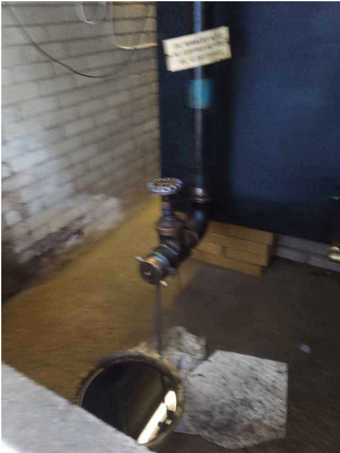
Location 03 - Oil Tank (2)
