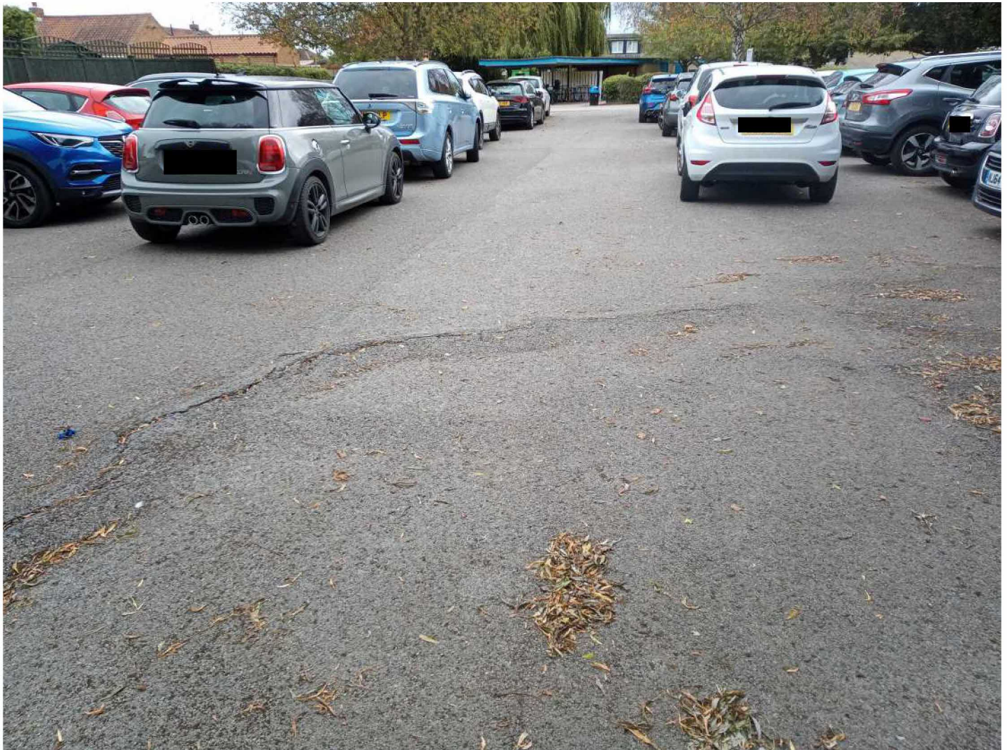
Location 17 facing North East - Staff car park and surface cracking
