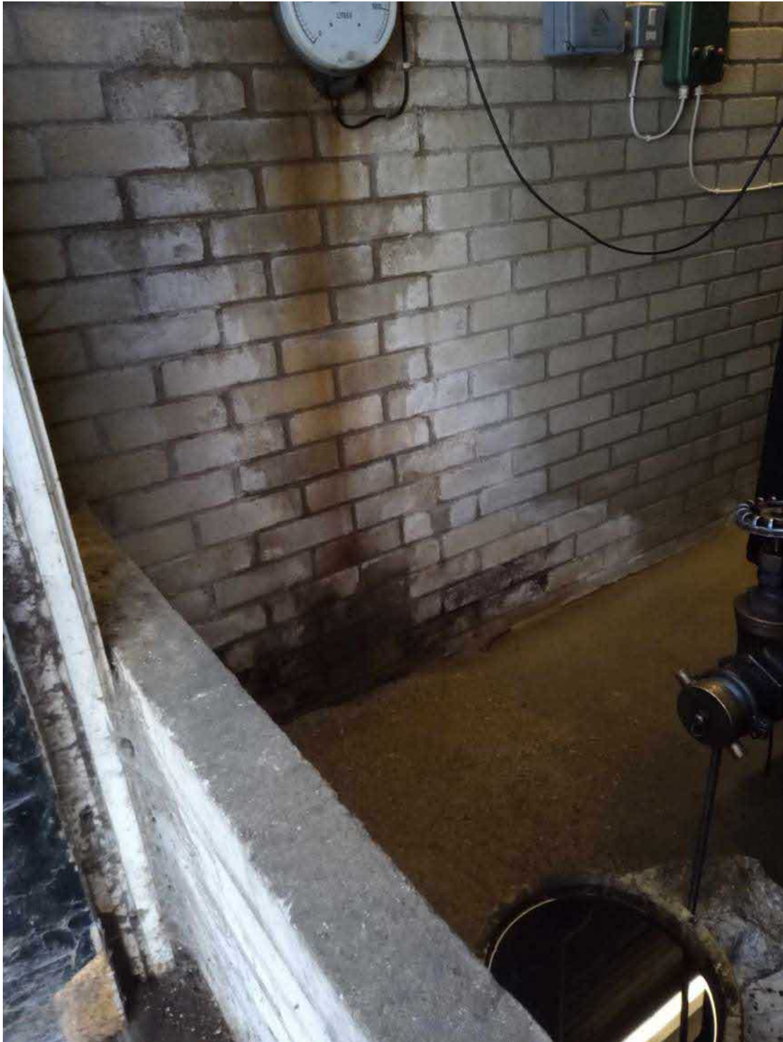
Location 03 - Oil Tank (1)
