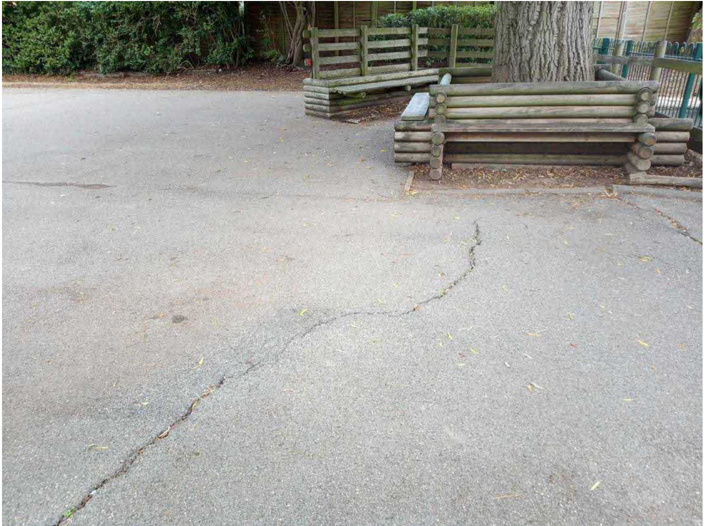
Location 16 facing North - Tarmac cracking radiating from tree
