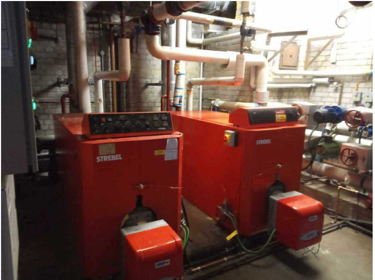
Location 18 - Inside the Boiler Room (3)
