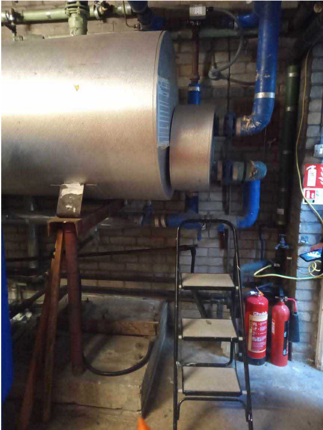
Location 18 - Inside the Boiler Room (1)
