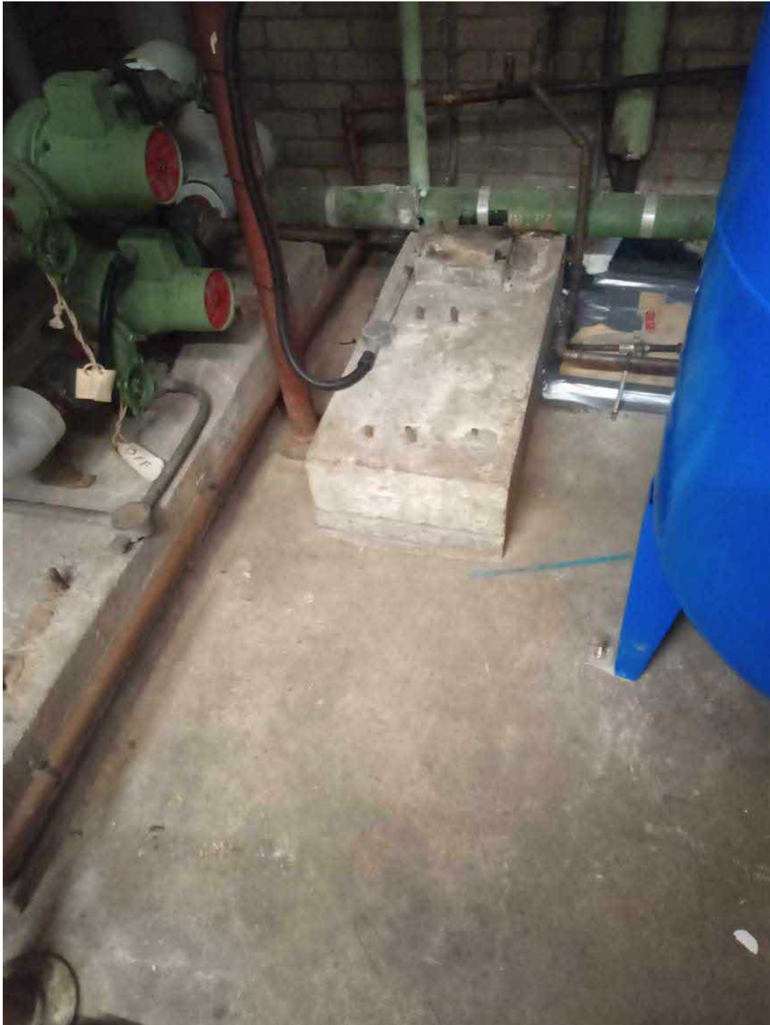
Location 18 - Inside the Boiler Room (2)
