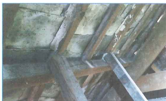
Most of the slate roofs were unlined to the inside
