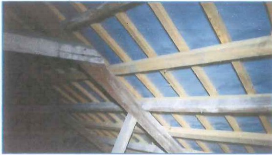
The northern pitch of the southern roof was lined with a breathable membrane
