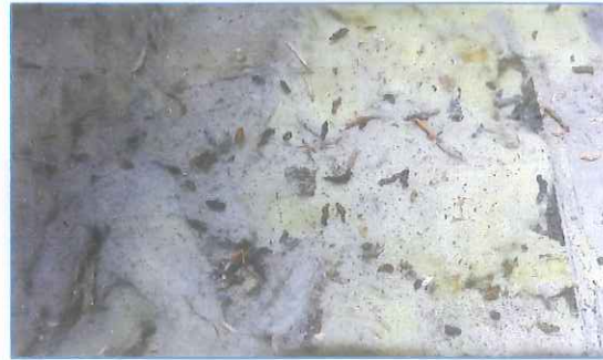
Accumulation of Long-eared bat droppings in the roof void beneath the southern roof
