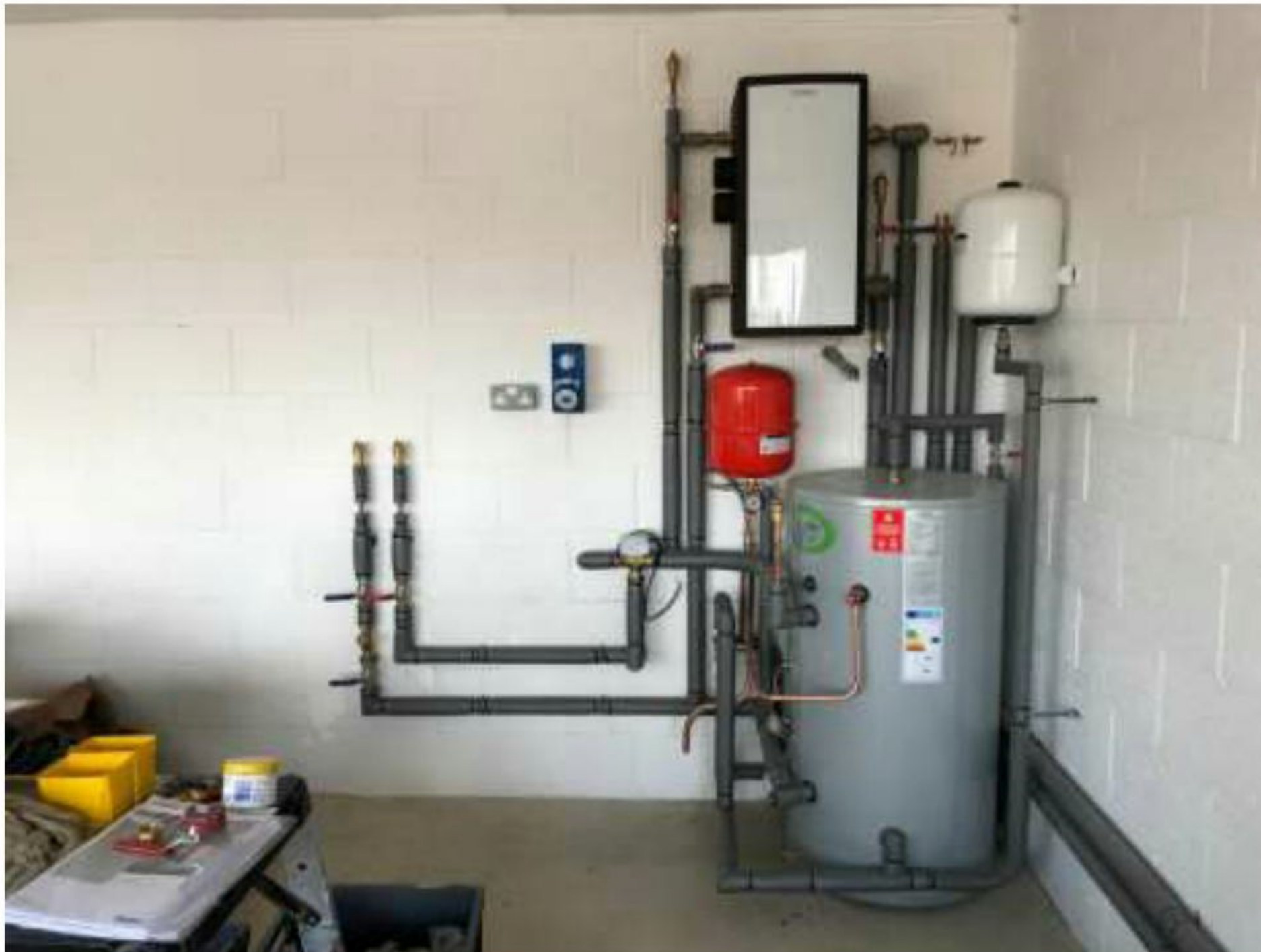
Typical internal works for an air source heat pump installation
