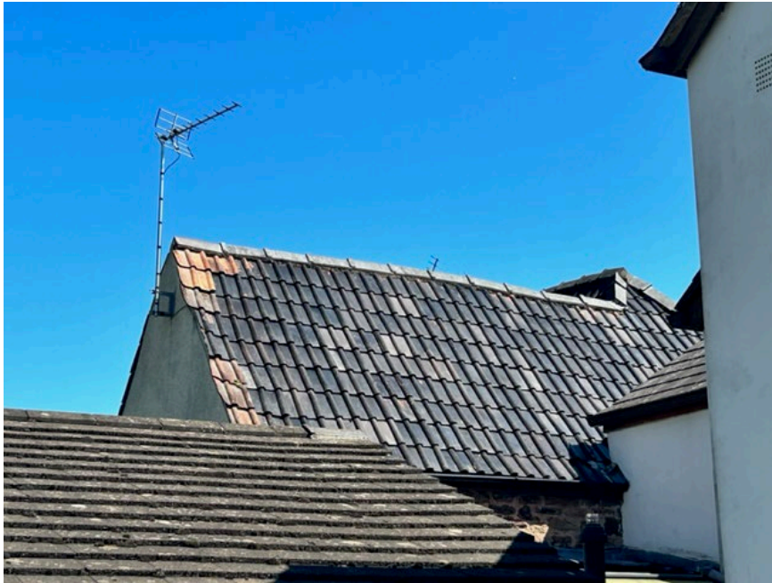
Photo 3: View of the side of the house / roof from the unnamed lane.
