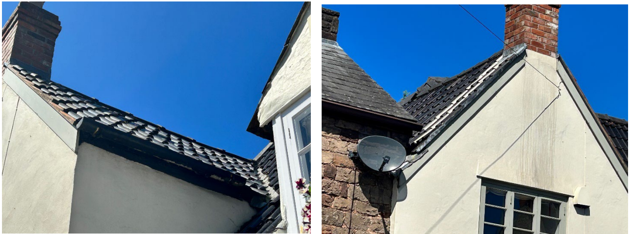
Photo 1 & 2: View of the front of the house (location of the proposed tile replacement) from the street.
