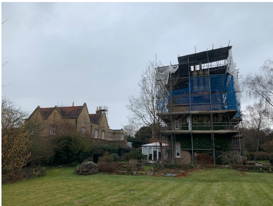
Figure 1: Gate House- from the garden looking north-west, showing the relationship to Hunsdonbury & the location of the existing modern conservatory- proposed to be demolished
