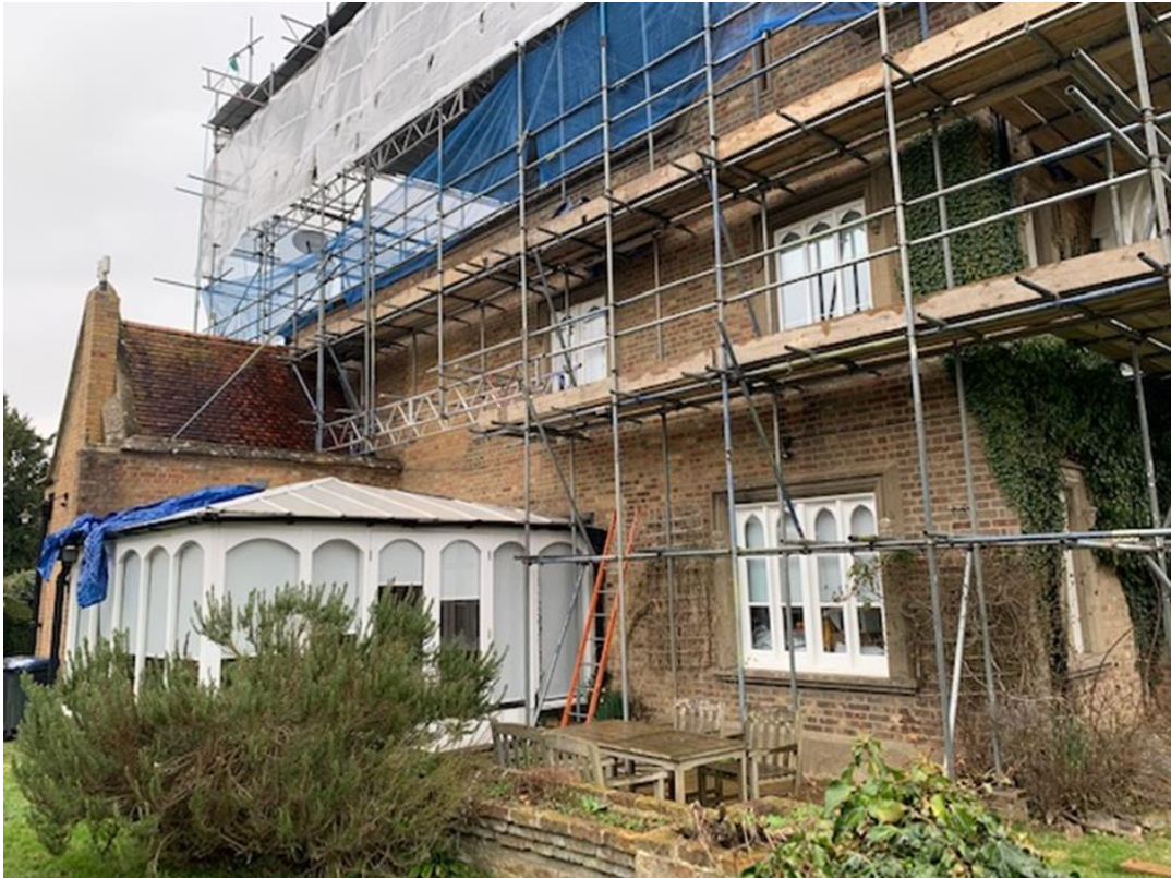
Figure 2: Gate House- from the garden looking north- the awkward relationship of the ungainly modern conservatory to the house
