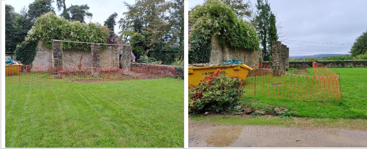
Photos showing the free-standing stone piers to the west of the Implement Shed (NB Orange net fence was temporarily installed during dismantling work)
