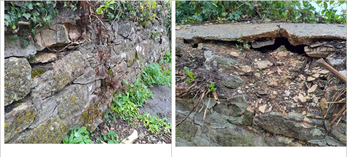
Close-up views of boundary wall showing current condition of 6m section that required re-building
