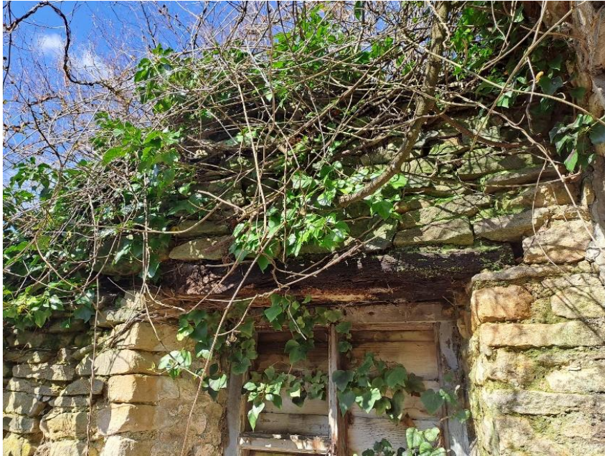
North wall (internal) showing unstable masonry and decayed window lintels
