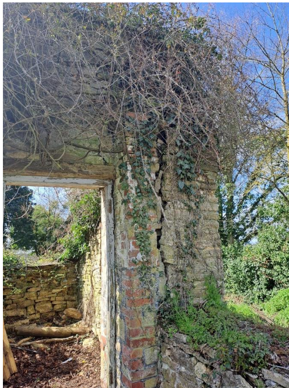
Northern extension after initial vegetation clearance showing large crack
