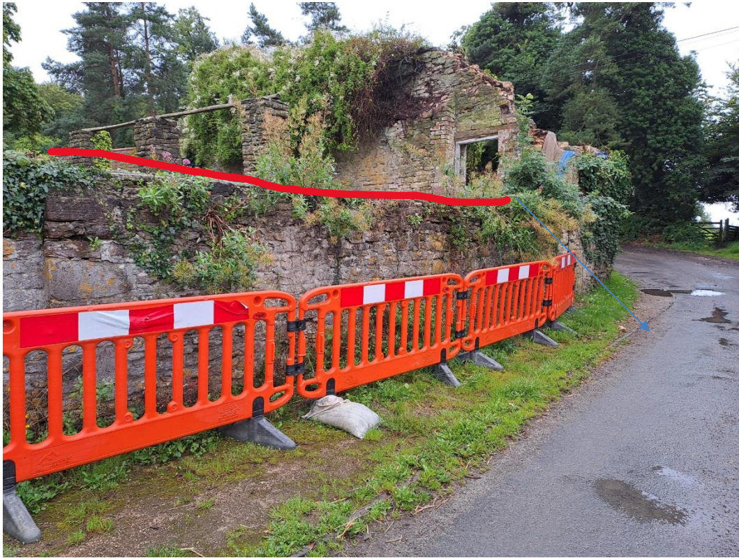
6m section of boundary wall that needs rebuilding (roadside view)
