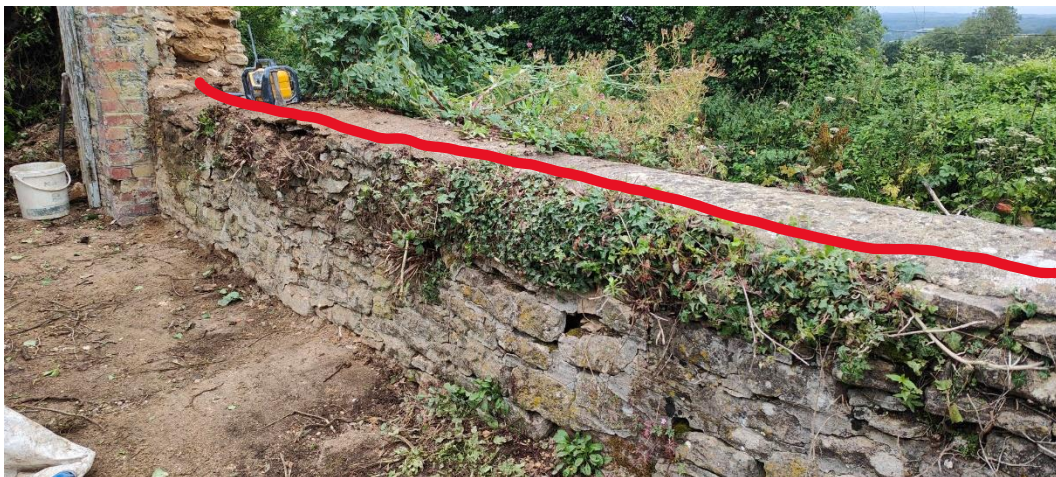
6m section of boundary wall that needs rebuilding (garden view)
