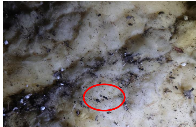
Photograph 15: Bat droppings in roof void.
