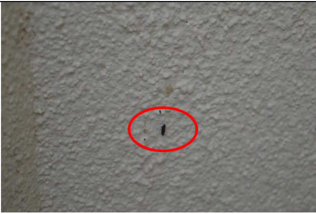
Photograph 12: View of bat dropping on external walls on north facing elevation.
