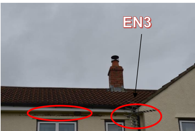
Photograph 5: View of the southern elevation EN3 and house martin nests.
