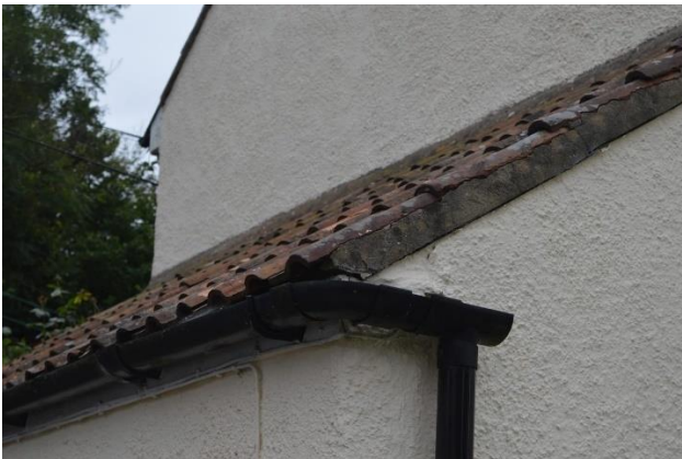
Photograph 3: View of the lean-to section attached to the main house on the northern elevation.
