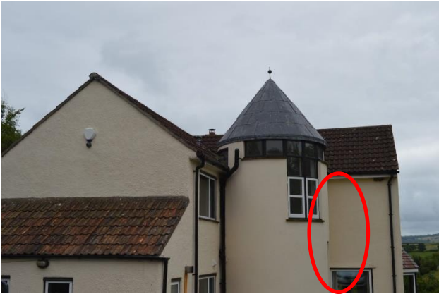
Photograph 1: View of the northern elevation of the house (location of bat droppings found stuck on the walls is circled in red).
