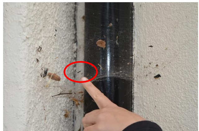
Photograph 12: Bat droppings in cobweb on the eastern facing elevation of the house.
