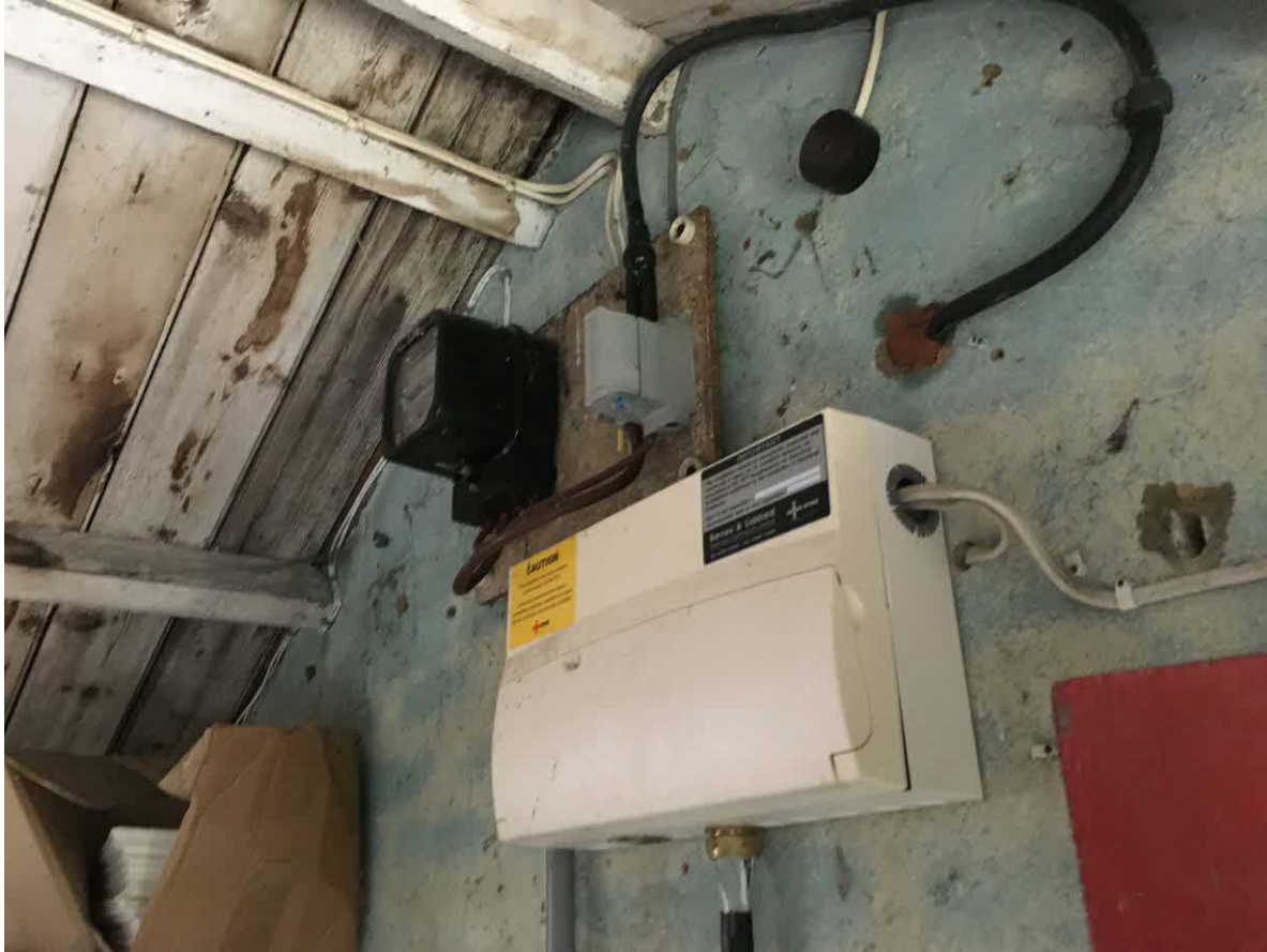
Outdated electrical supply
