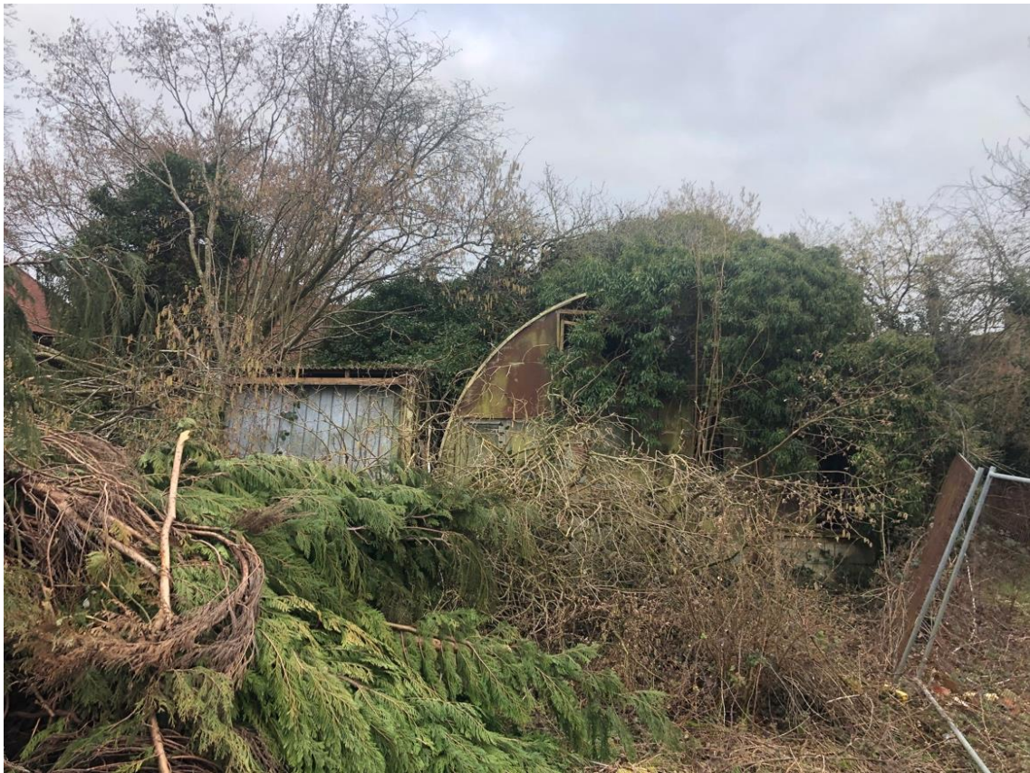
Photo 4: Building 8 on the right with the semi-circular roof, with a thick ivy cover suitable for nesting birds
