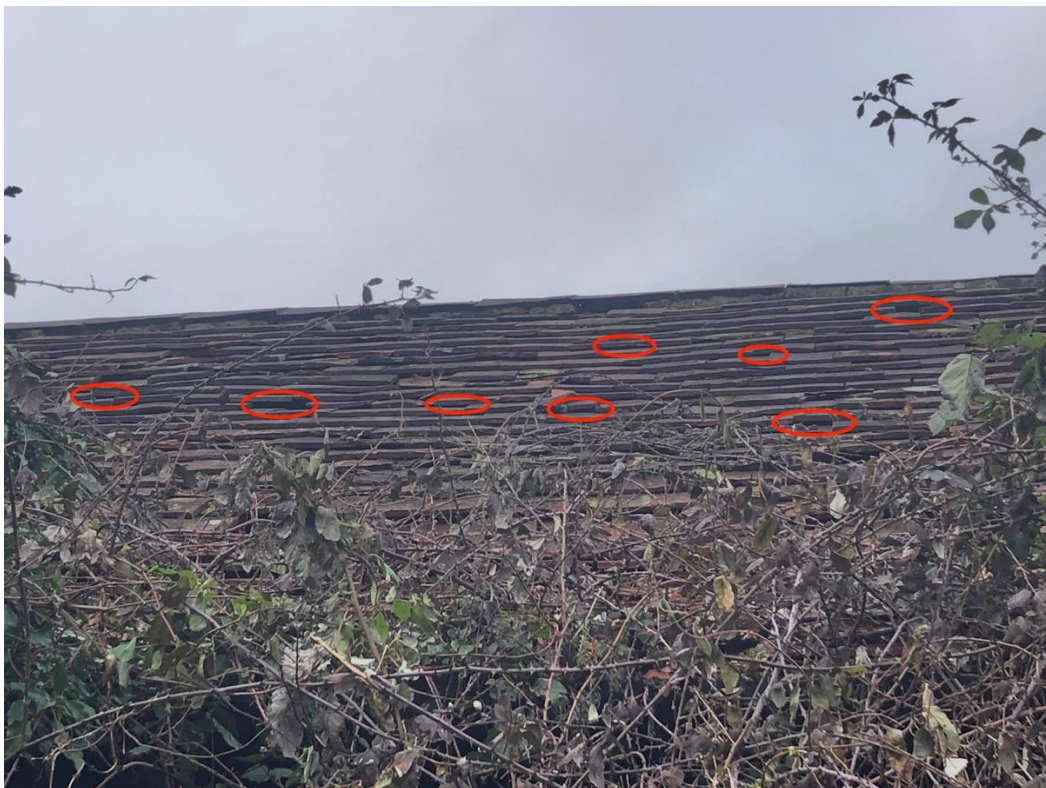
Photo 6: South-facing roof of one-storey dwelling (building 5), with some of the gaps under roofing tiles circled (red)
