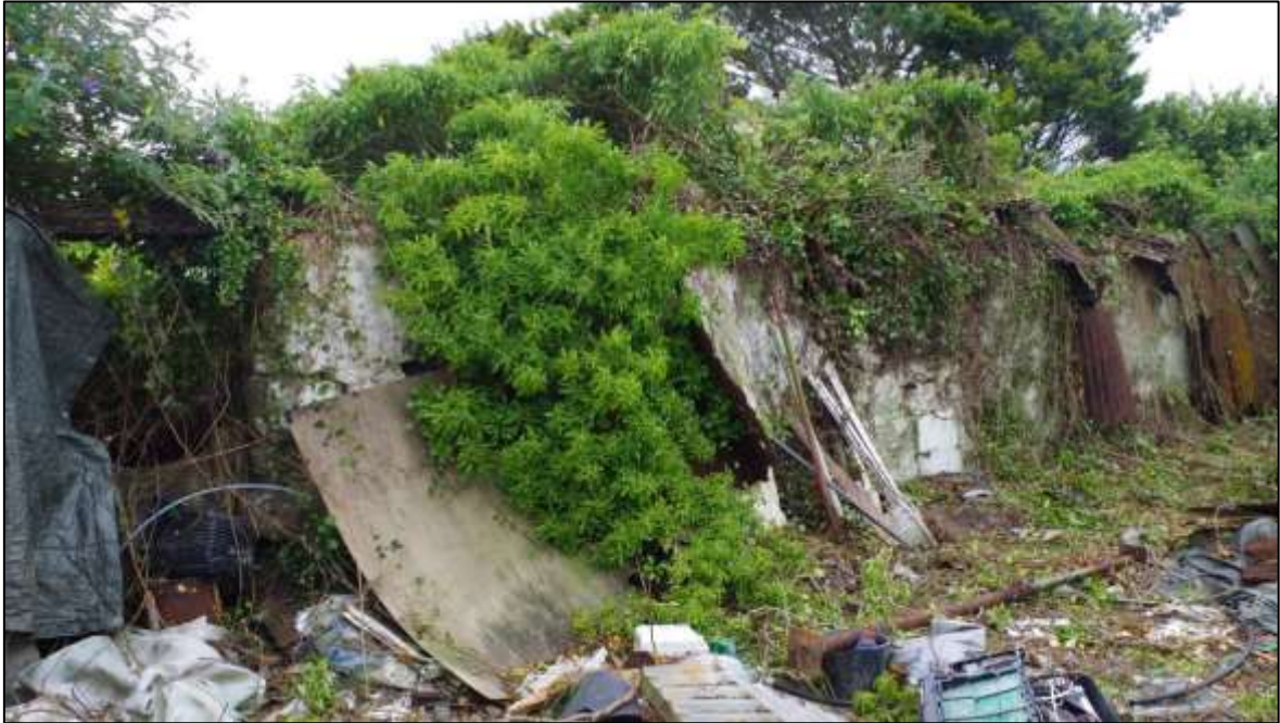
FIGURE 14: A DOOR AND TWO WINDOWS WERE IDENTIFIED IN THE SOUTH-EAST ELEVATION; VIEWED FROM THE NORTH.
