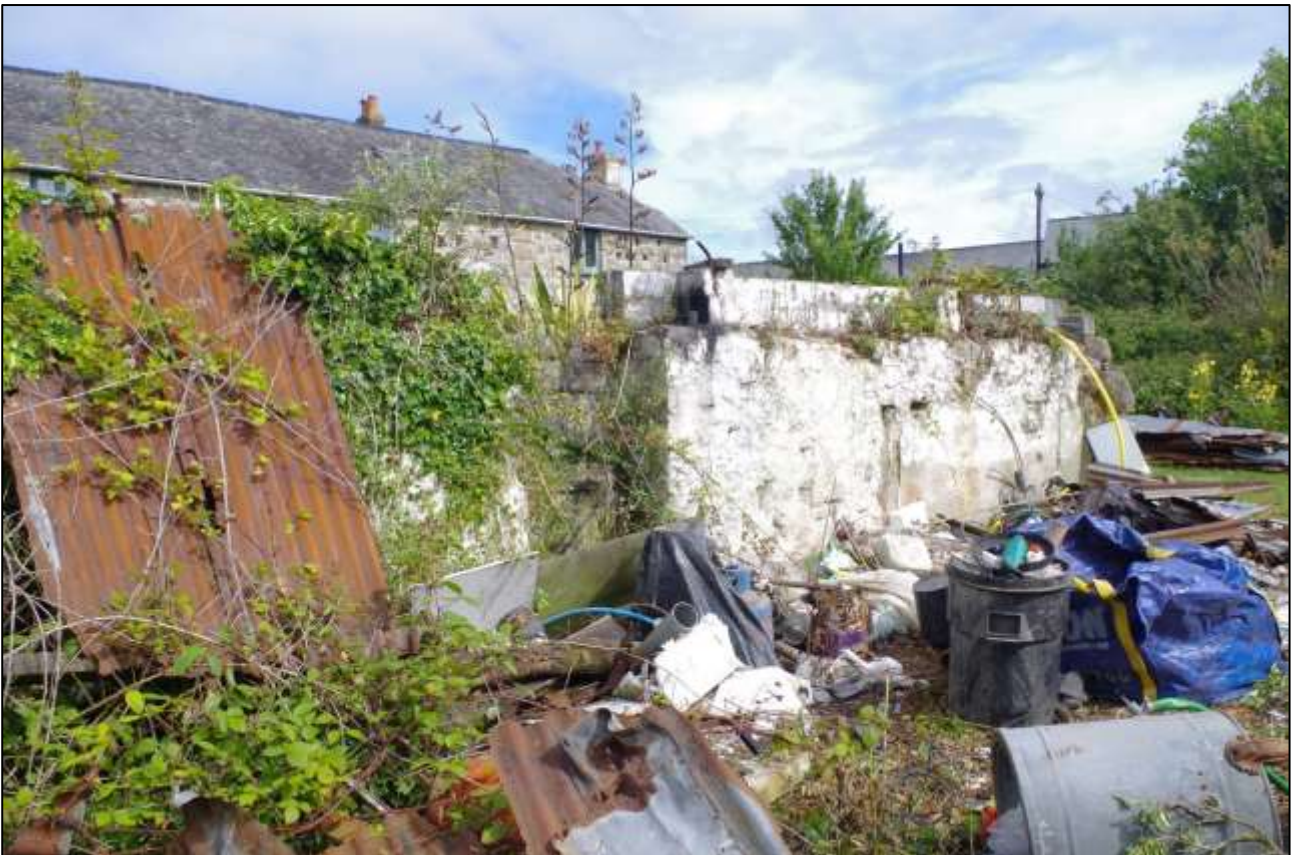
11. THE NORTH END OF THE NORTH-WESTERN INTERNAL ELEVATION; VIEWED FROM THE SOUTH-EAST.
