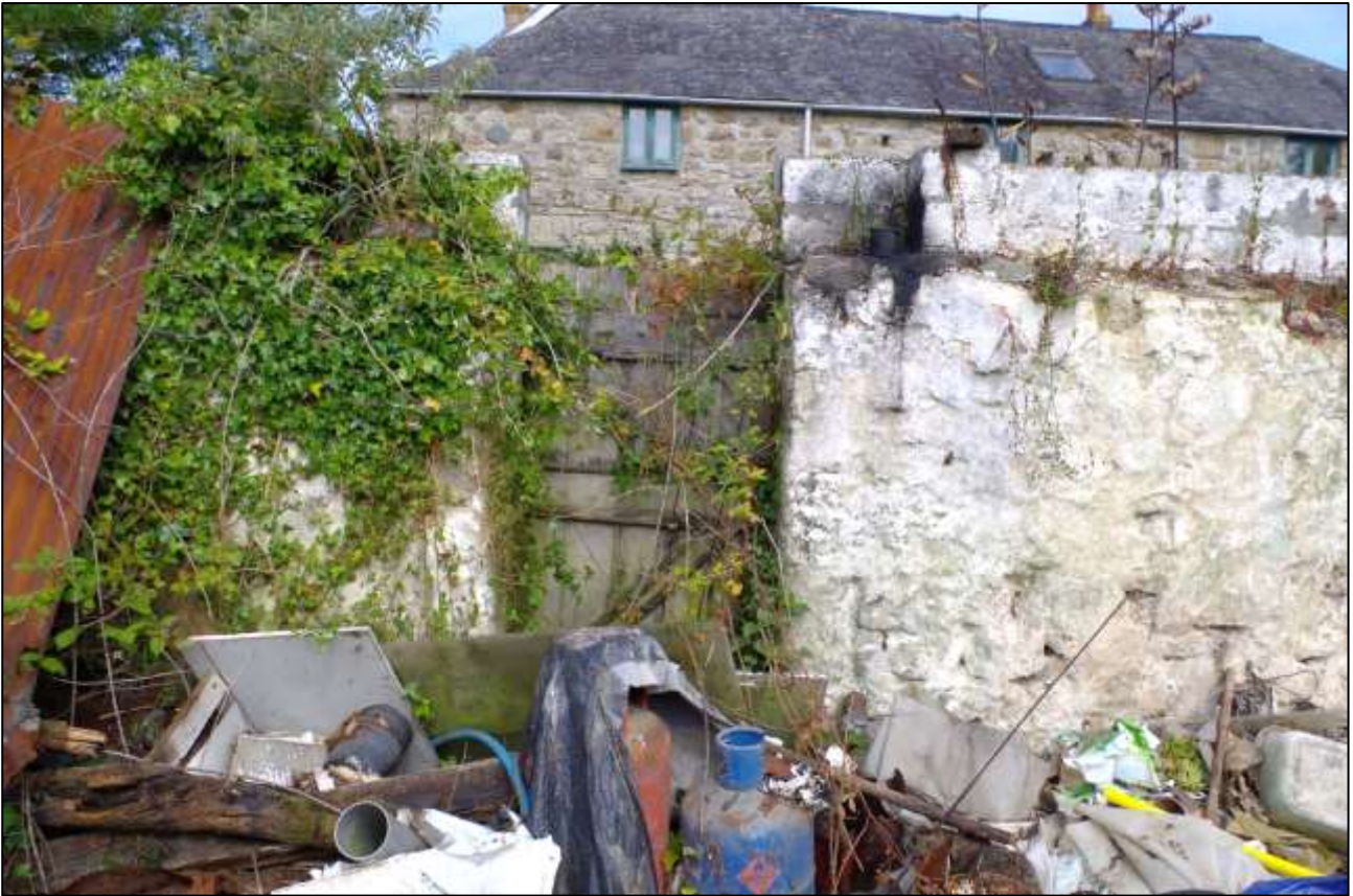
12. POSSIBLE LATER FORCED DOORWAY TO THE NORTH-WEST ELEVATION; VIEWED FROM THE SOUTH-EAST.
