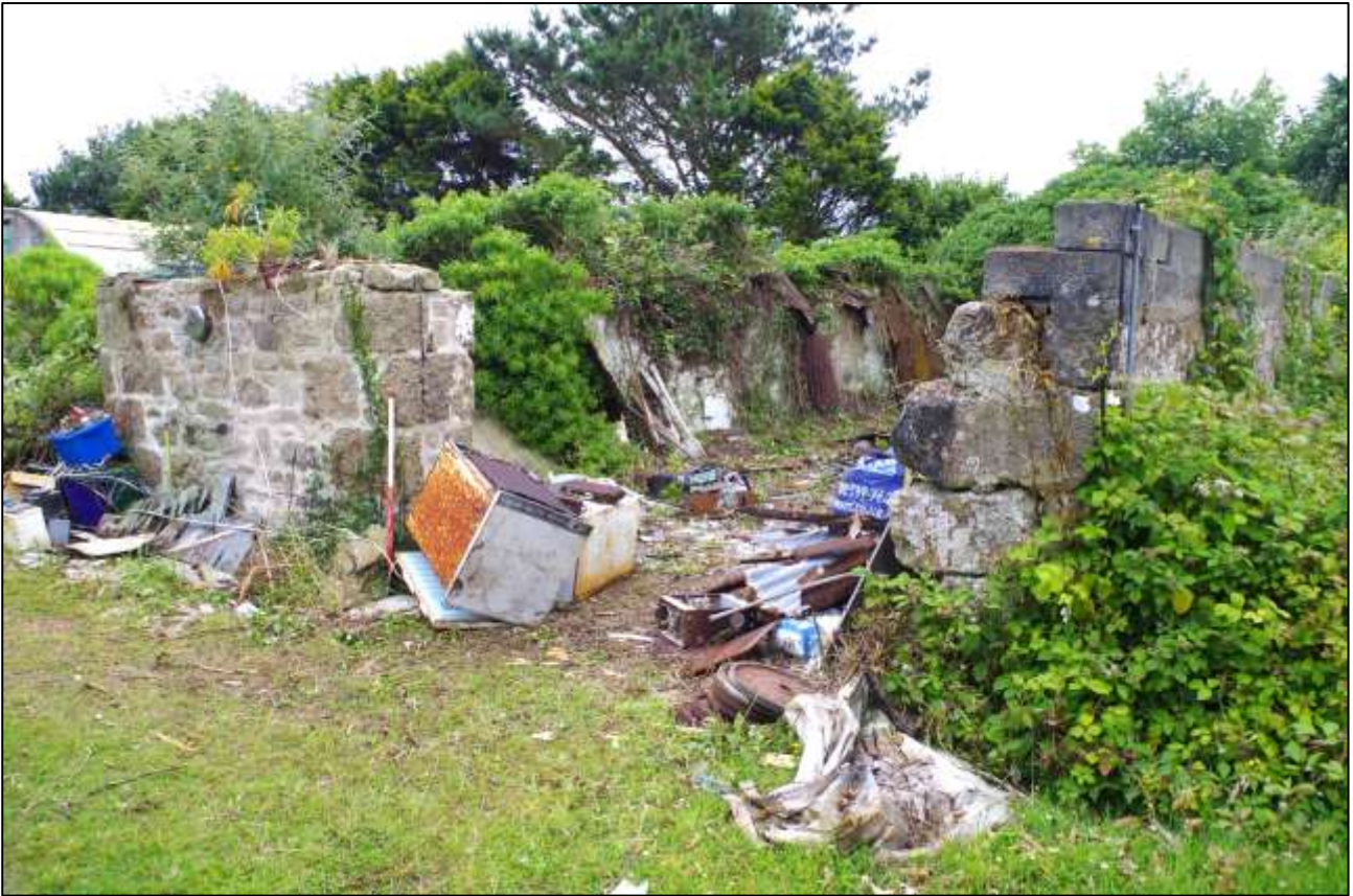
6. THE NORTH-EAST GABLE ELEVATION OF THE RUINED BARN; VIEWED FROM THE NORTH (1M SCALE).
