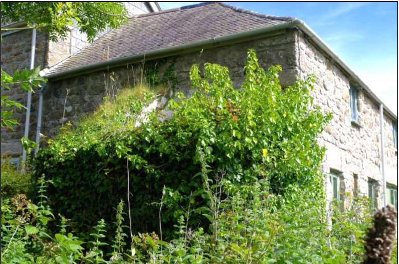
15. THE SMALL DERELICT LEAN-TO AT THE SOUTH END OF THE FORMER GRANARY; VIEWED FROM THE SOUTH.
