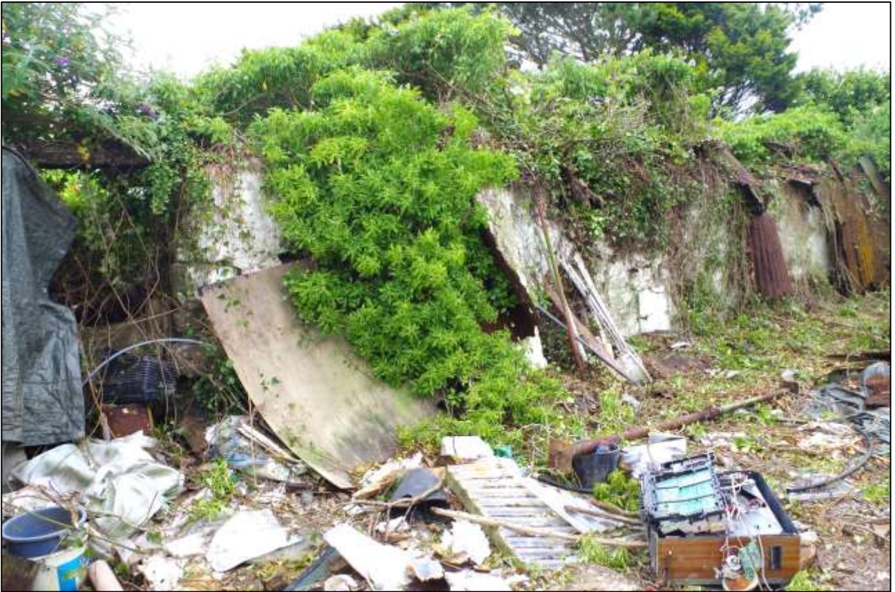
8. THE INTERNAL SOUTH-EAST ELEVATION, THE PARTIALLY-BLOCKED DOORWAY TO LEFT; VIEWED FROM THE NORTH-WEST.
