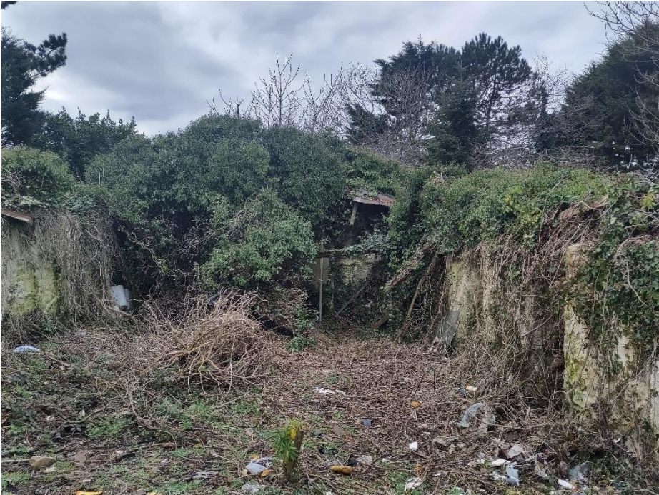
Photo 10: ruinous stone barn showing interior and dense Ivy on wall-tops.
