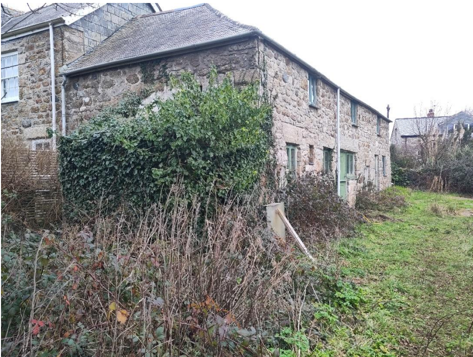
Photo 8: collapsed lean-to on southern elevation of the Granary supporting dense Atlantic-ivy growth.
