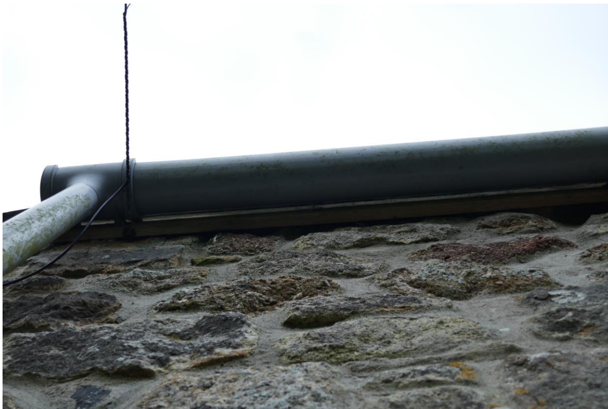
Figure 4. Gap behind fascia on north side of the granary, suitable for roosting bats.
