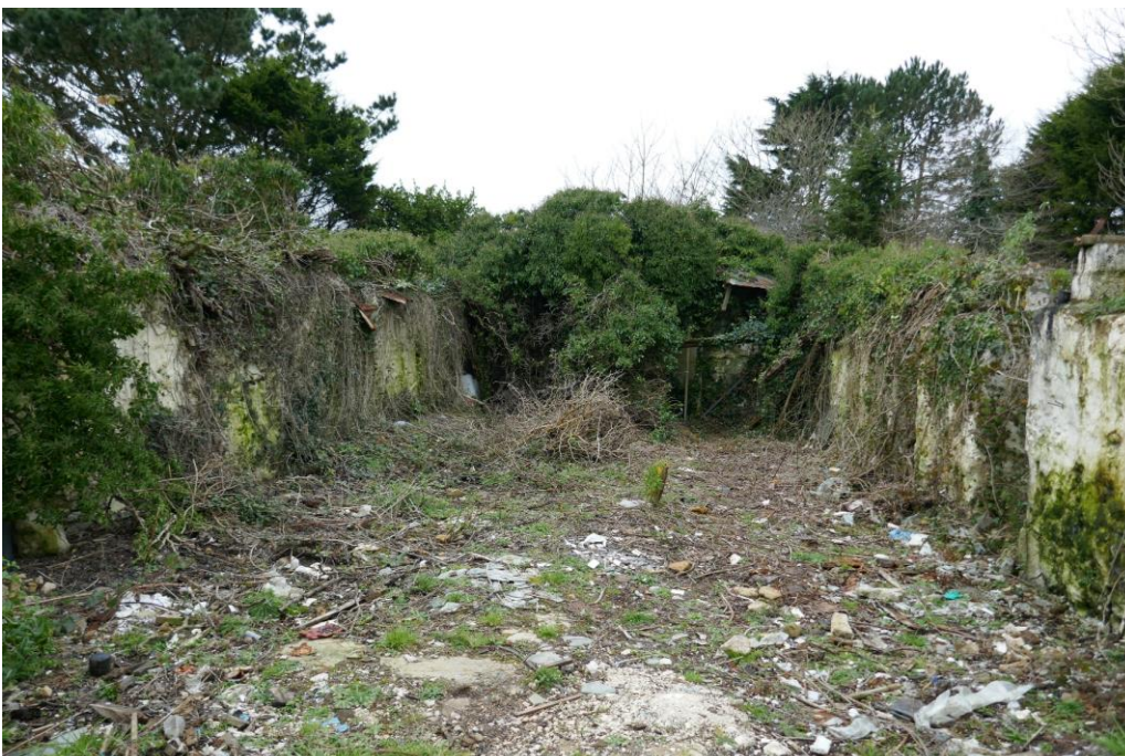
Figure 11. Interior of collapsed barn.
