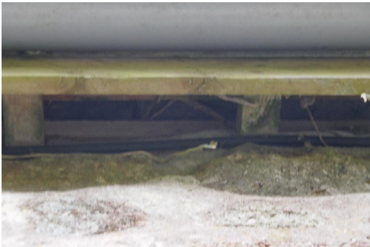
Figure 5. Open gap on the southern gable, leading into the roof void.
