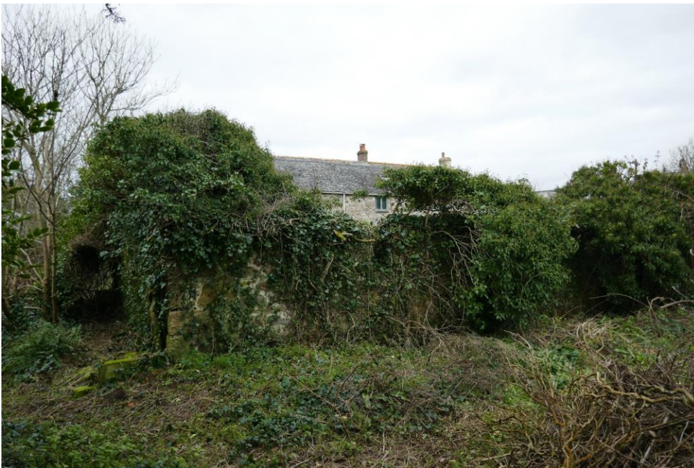
Figure 10. Eastern aspect of the collapsed barn, looking towards the granary.
