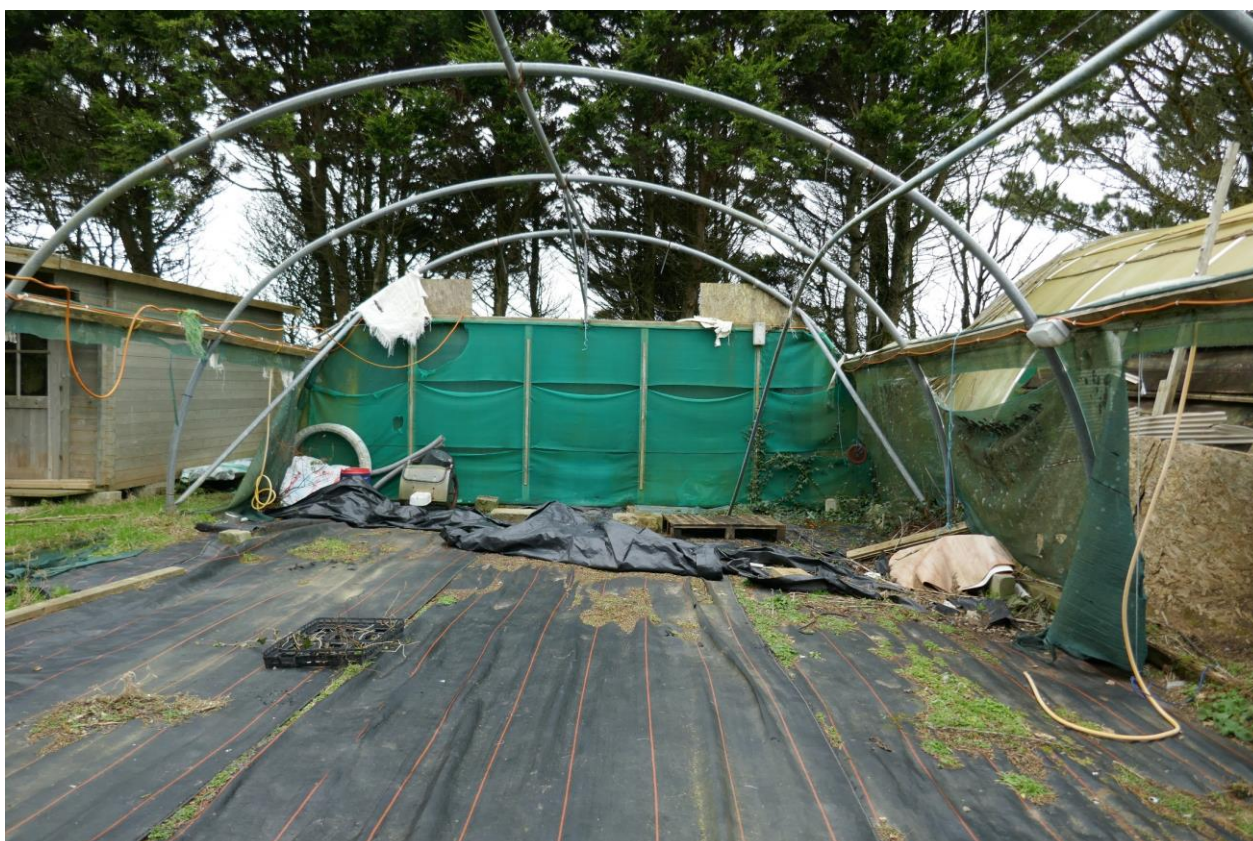
Figure 15. Remains of the polytunnel.
