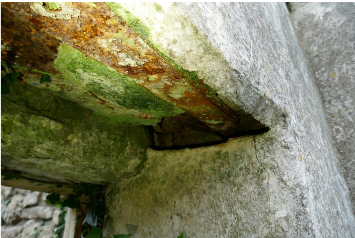
Figure 9. Recess leading into the stonework at the edge of the lean-to entrance.
