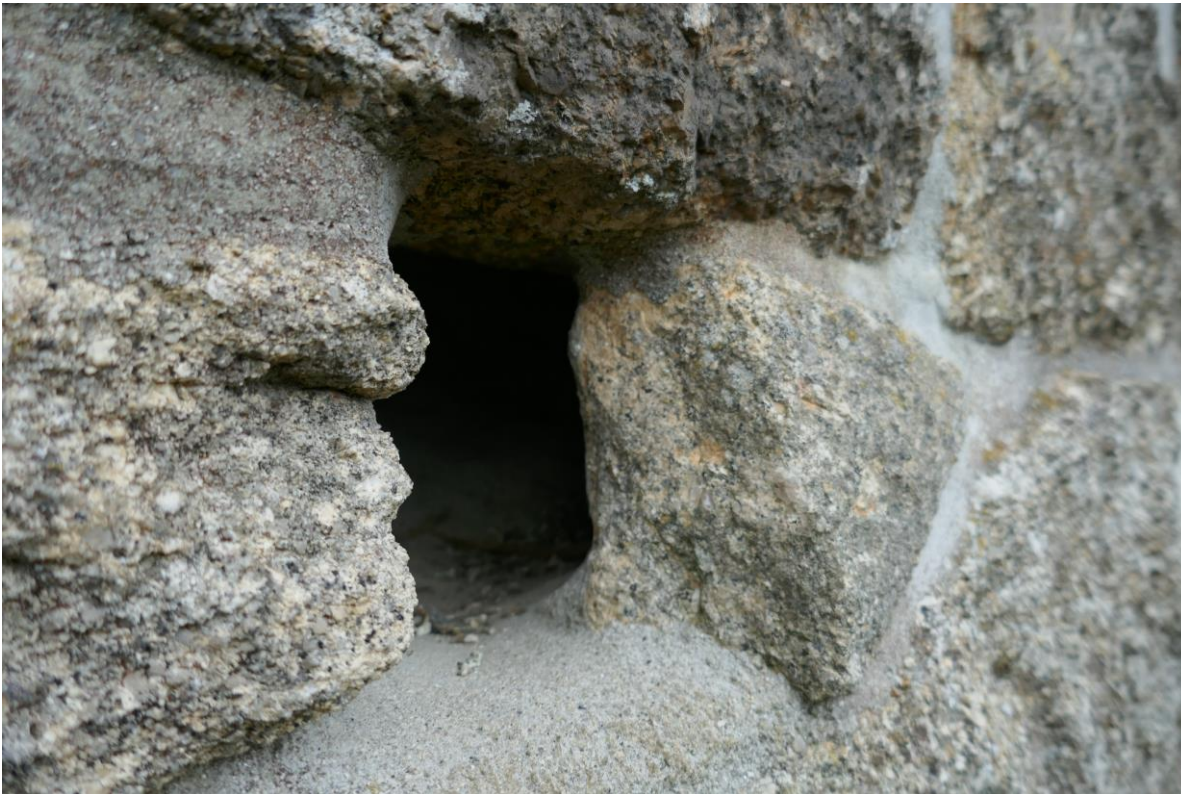
Figure 2. Close-up of one of the square holes in the eastern aspect of the building.
