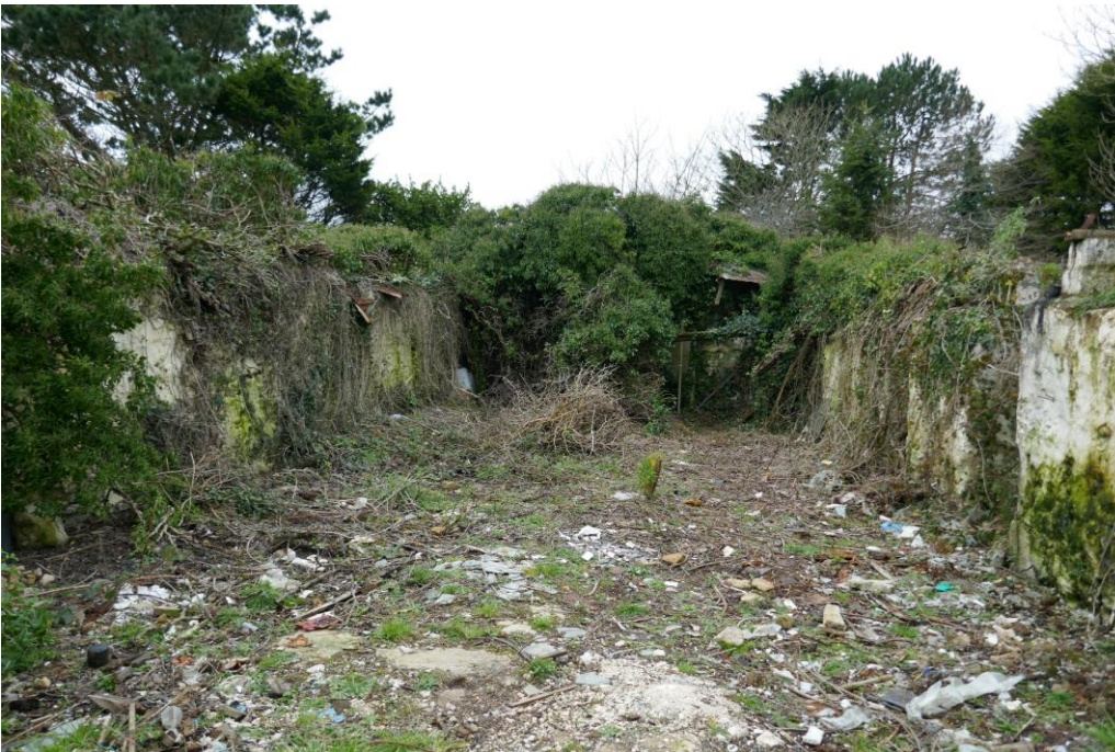
Figure 11. Interior of collapsed barn.
