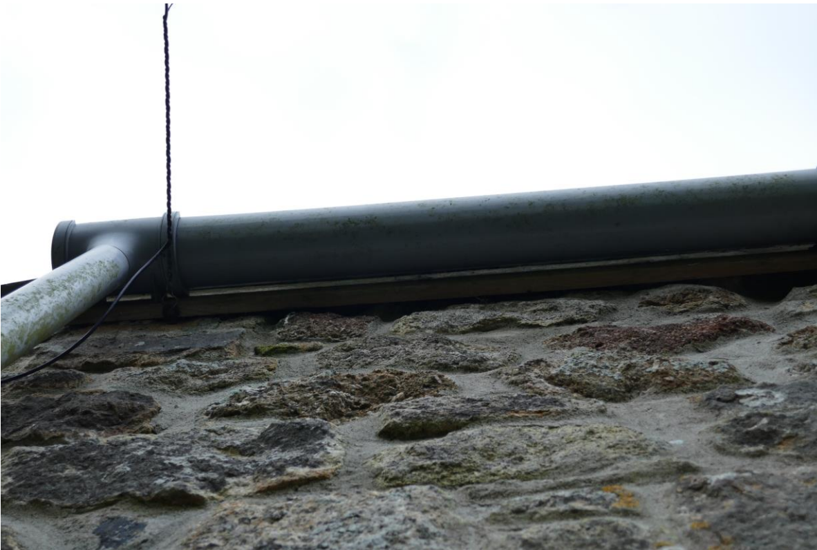
Figure 4. Gap behind fascia on north side of the granary, suitable for roosting bats.
