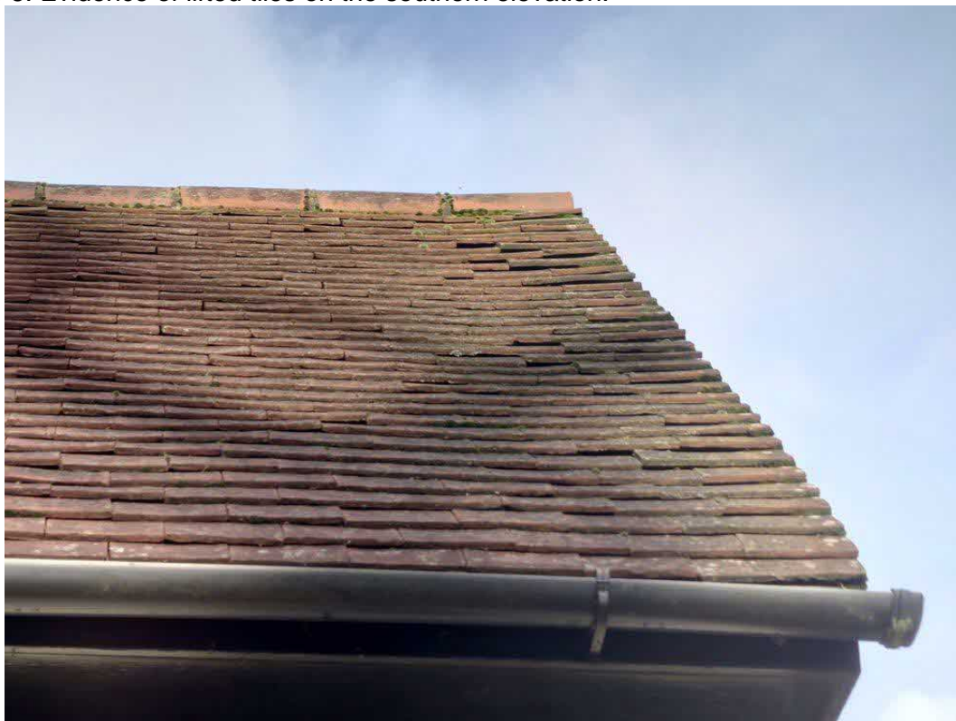
Plate 5: Evidence of lifted tiles on the southern elevation.
