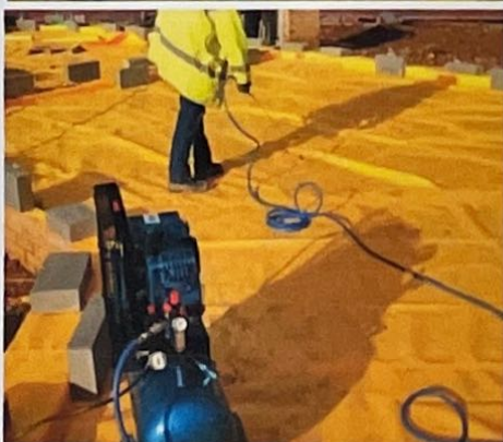
Photograph 5: Showing the process of Air Lance testing in progress to verify the quality of the welded seams along gas membrane joints. Check top hat is sealed to membrane and pipework.
