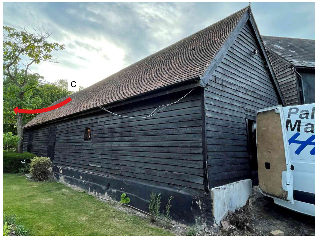
Two common pipistrelles emerged from gaps under roof tiles on the southern elevation of the pitched roof at 16 and 18 minutes after sunset (Roost C).
