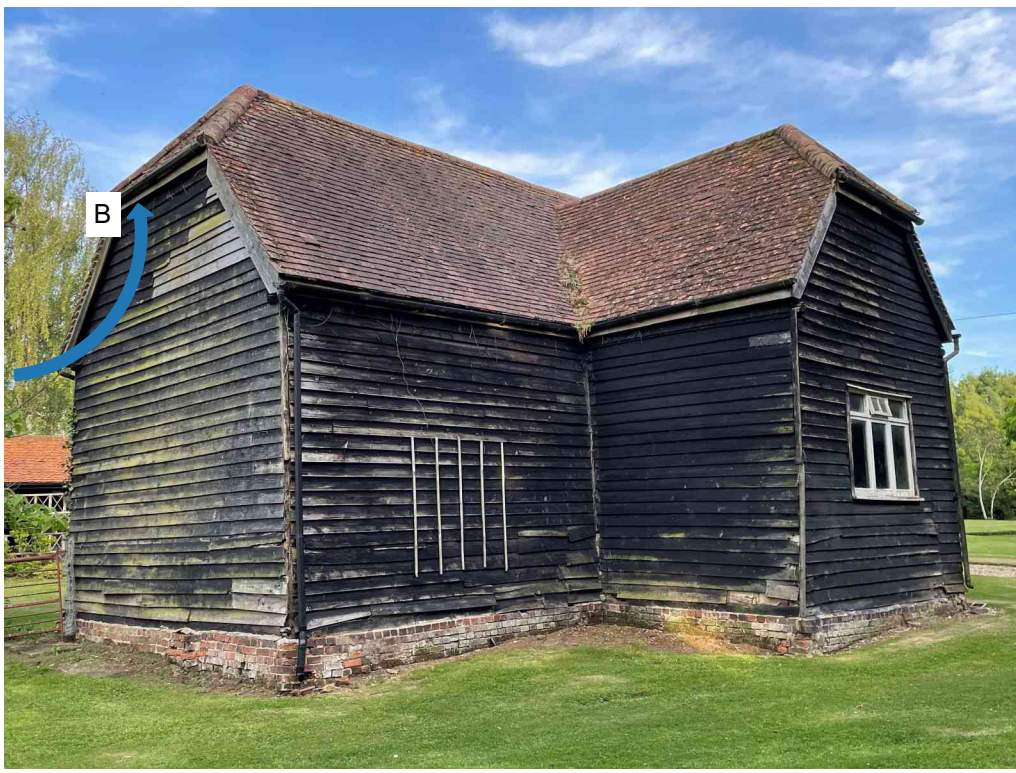
Two brown-long eared bats returned to roost via a gap under the fascia on the northern gable end at 61 and 78 minutes after sunset (Roost B).
