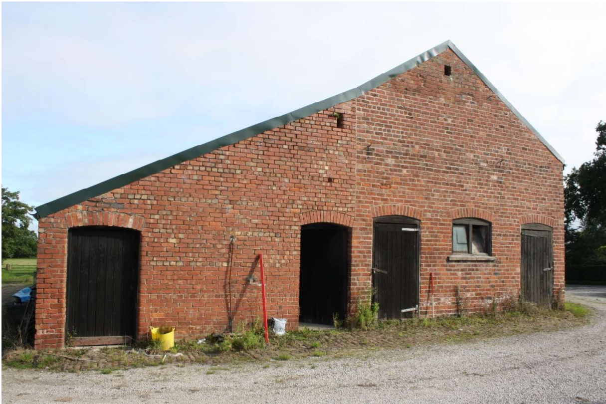
Plate 2 South elevation of the barn, facing northeast. Outshut to the east is a later addition.
