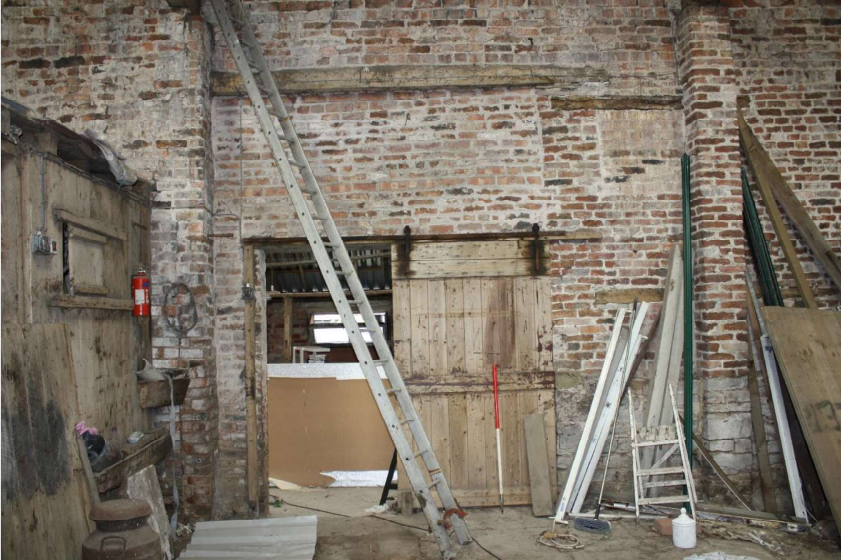
Plate 24 Modern replacement of the wagon door in the west elevation, facing west.
