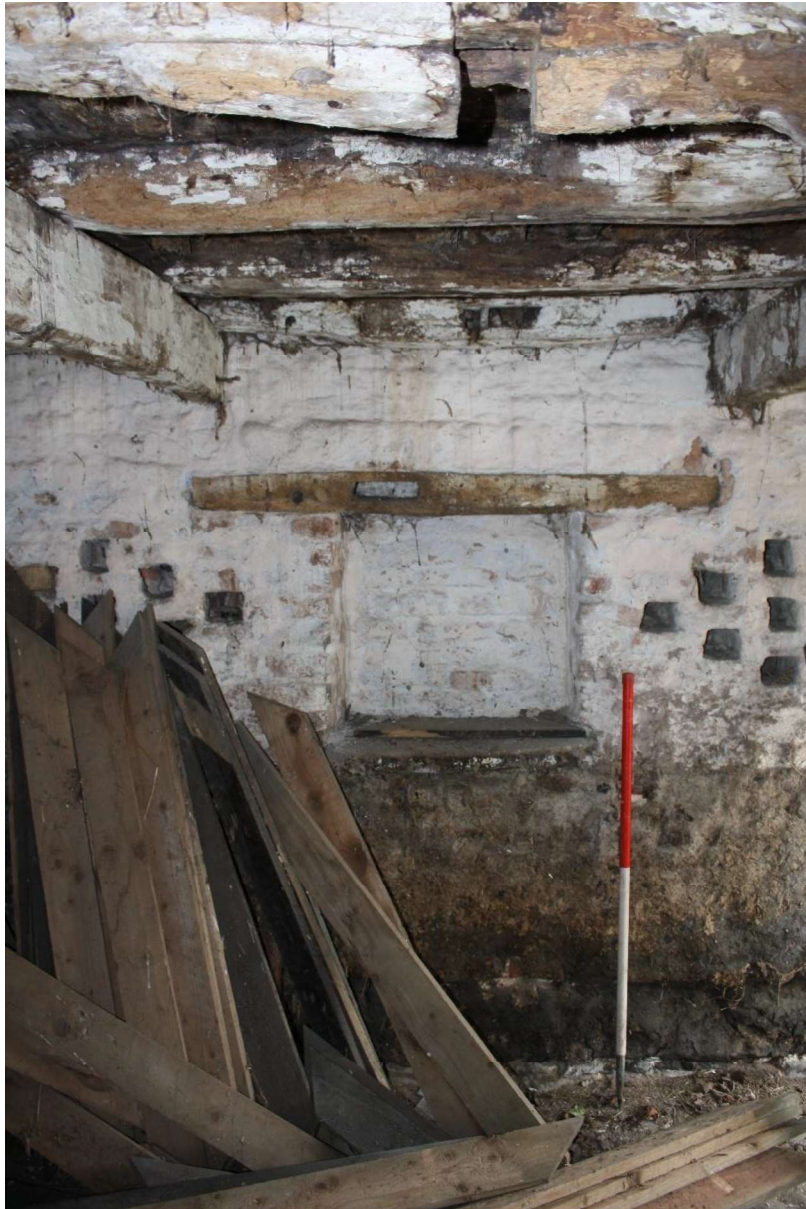
Plate 29 Blocked aperture and ventilation slots in the west elevation of the cowhouse.
