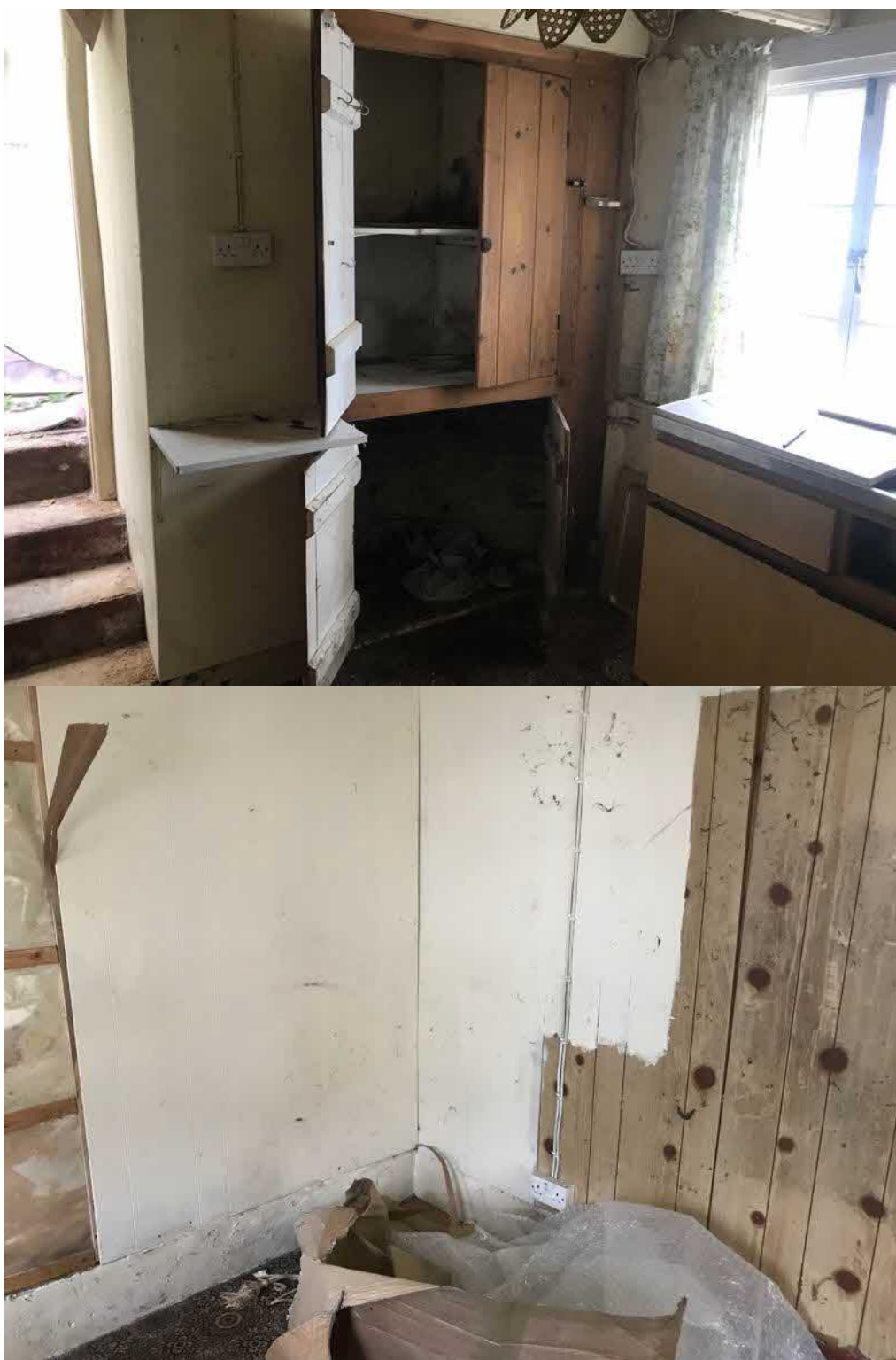
Figure 9: Details of the south eastern and north western corners of the kitchen wing
