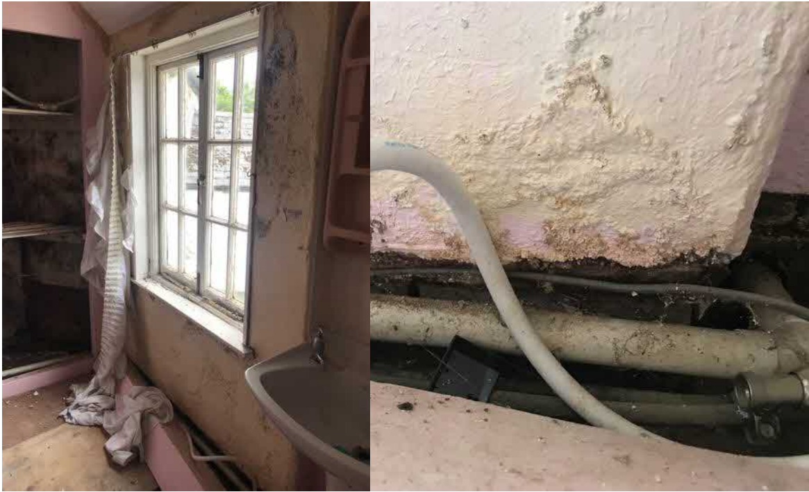
Figure 17: Composite view showing severe mould, blistering paint and plaster, and ad hoc plumbing
