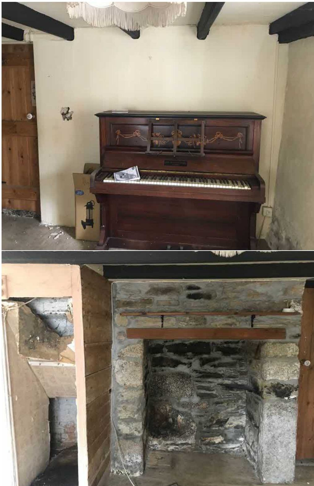
Figure 6: Views of the principal ground floor room of the cottage. Above: note battering-out of the wall, plus mould. Also note area of exposed gypsum plaster and battenning out of wall (this has been done throughout the ground floor).
