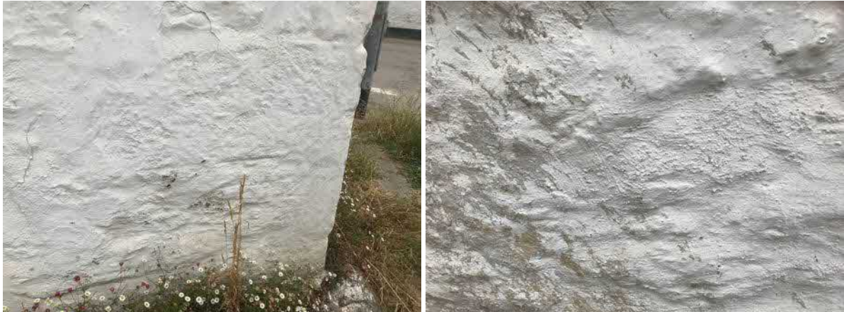
Figure 5: Details showing condition of exterior fabric
