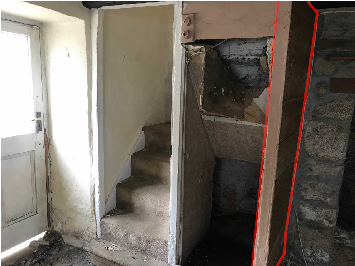
Figure 7: Detail view of staircase showing rot of staircase treads and risers, and with probable 19th century panelling section marked in red.
