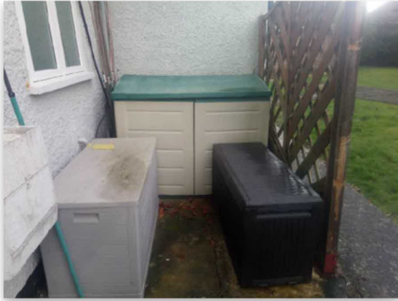
Fig 3.1: Storage boxes preventing access to MH
