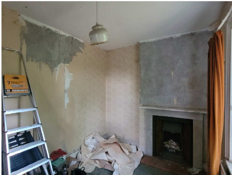
Existing reception room. Flue lined and living flame gas fire to be fitted.
