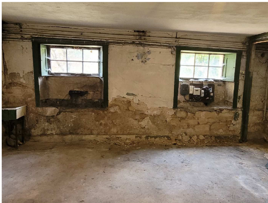
Dampness to basement and incoming electrical supply to right hand side
