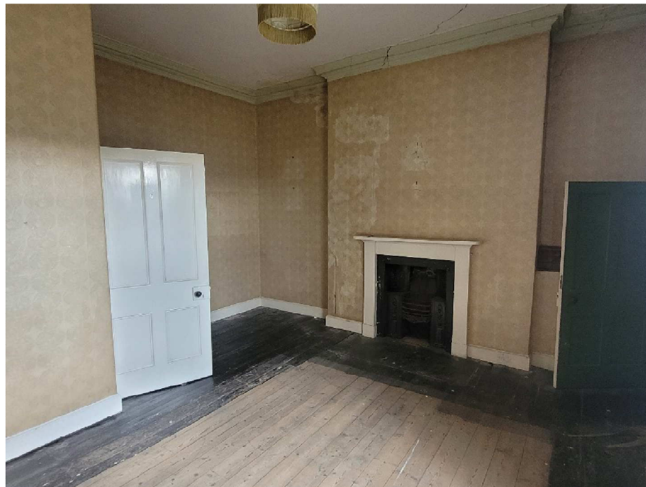
Bedroom 1. Alter partitions to form shower room. Reinststate coving. Line flue and fit living flame gas fire
