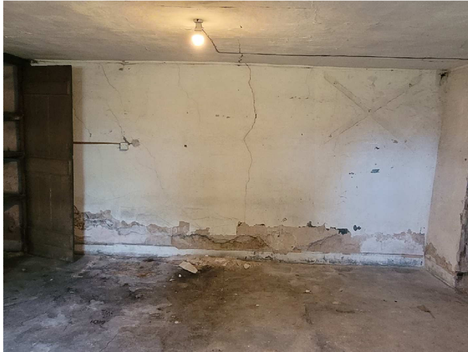
Dampness to basement
