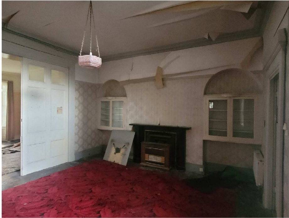
Existing dining room. Flue lined and living flame gas fire to be fitted.
