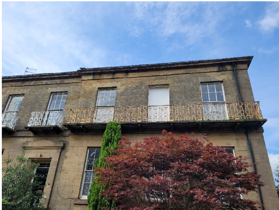
White board to dummy window to be replaced with dummy sash to match elsewhere
