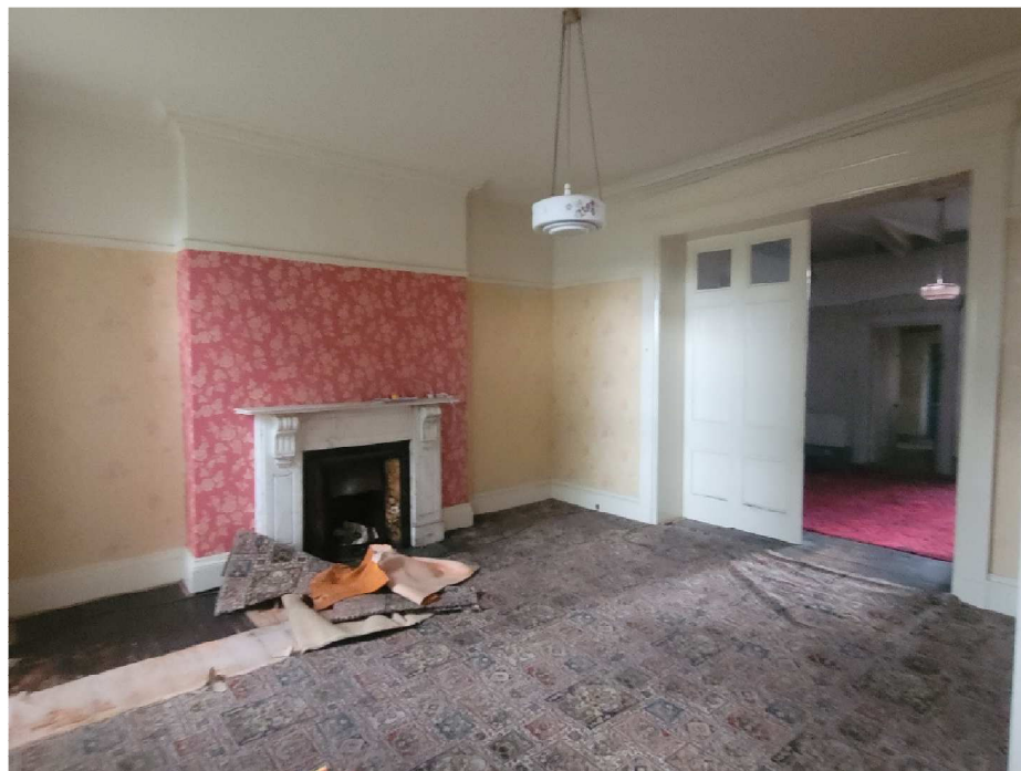
Existing living room. Flue lined and living flame gas fire to be fitted.
