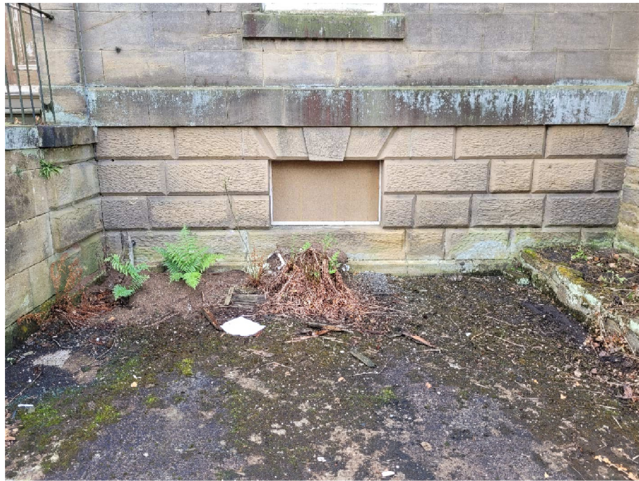
Basement window to be reinstated
