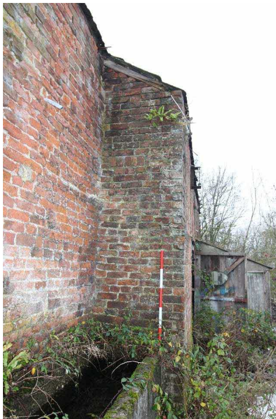
Plate 26: Scar of roof line on south-facing return wall. Facing north with 1m scale
