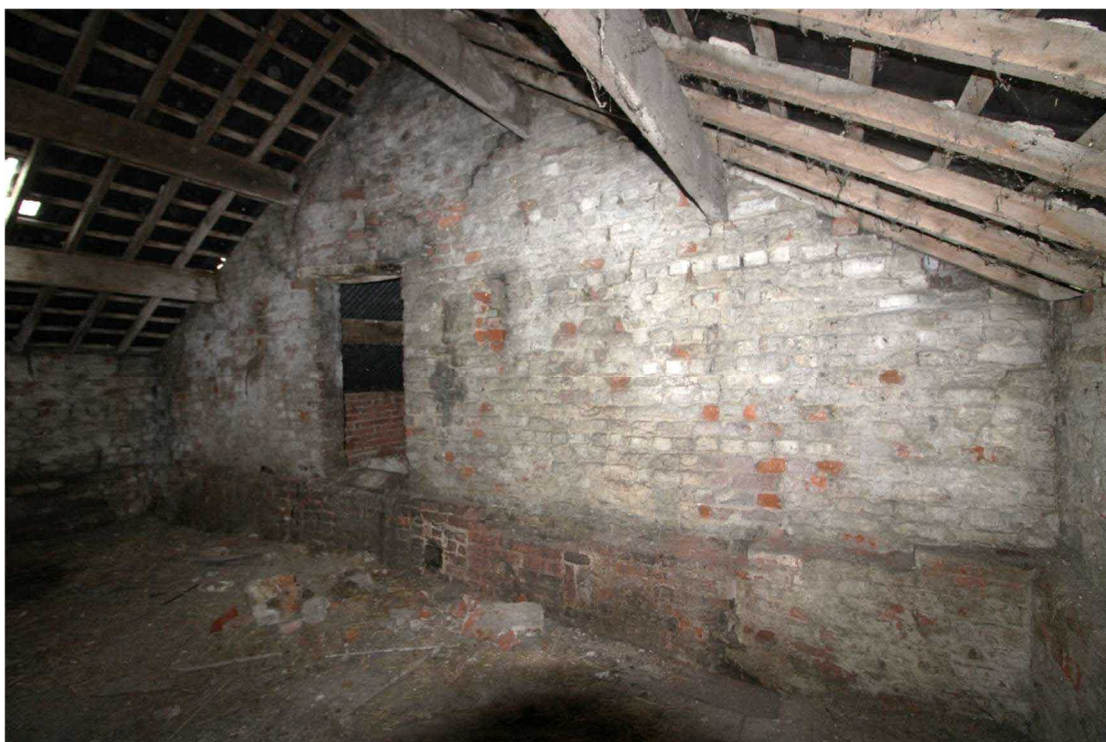
Plate 47: Southern gable at mezzanine level, facing south-east. Note the narrow brick ledge running across the southern, eastern and western walls
