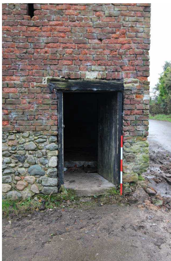
Plate 15: Entrance to northern byre at western end of northern elevation. Facing south, with 1m scale
