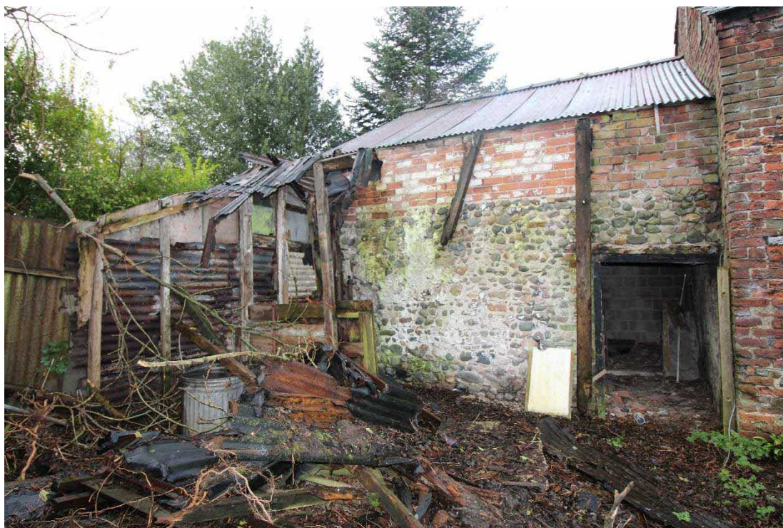
Plate 32: Eastern elevation of Southern extension, facing west
