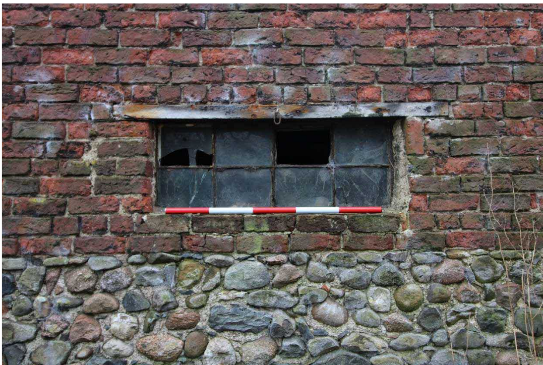
Plate 18: Window at centre of northern gable elevation. Facing south, with 1m scale
