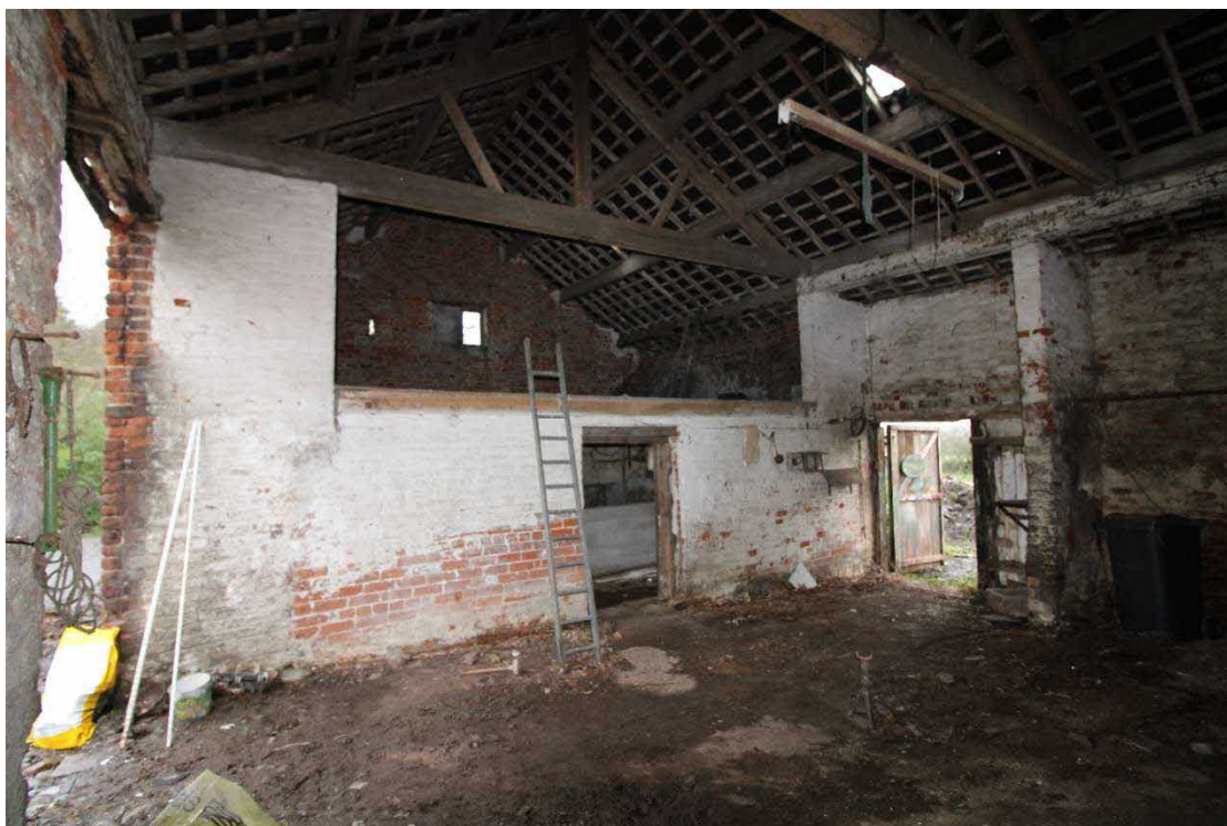
Plate 44: Threshing floor, showing vertical construction joint at the base of the wall to left of frame
