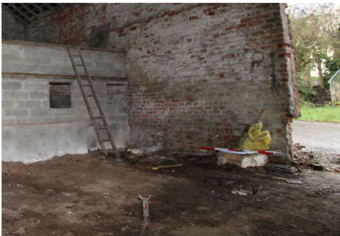
Plate 43: Threshing floor, facing south-west with concrete plinths projecting from the base of the wall
