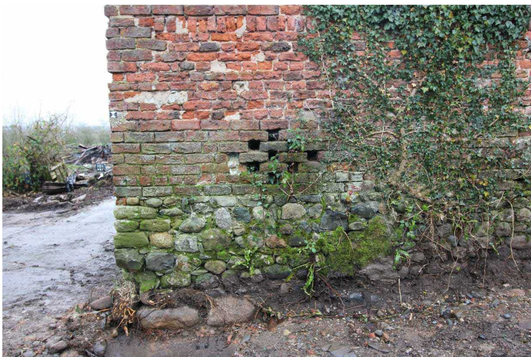
Plate 11: Diamond pattern ventilation loop at northern end of western elevation
