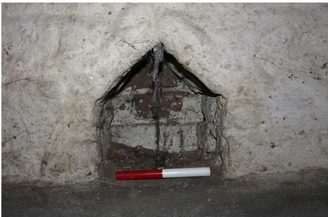
Plate 37: Triangular-headed niche to west of blocked doorway. Facing north with 0.2m scale
