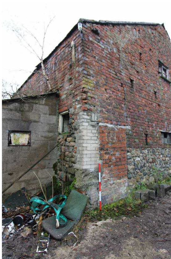
Plate 17: Blocked doorway at eastern end of northern elevation. Facing south-west with 1m scale
