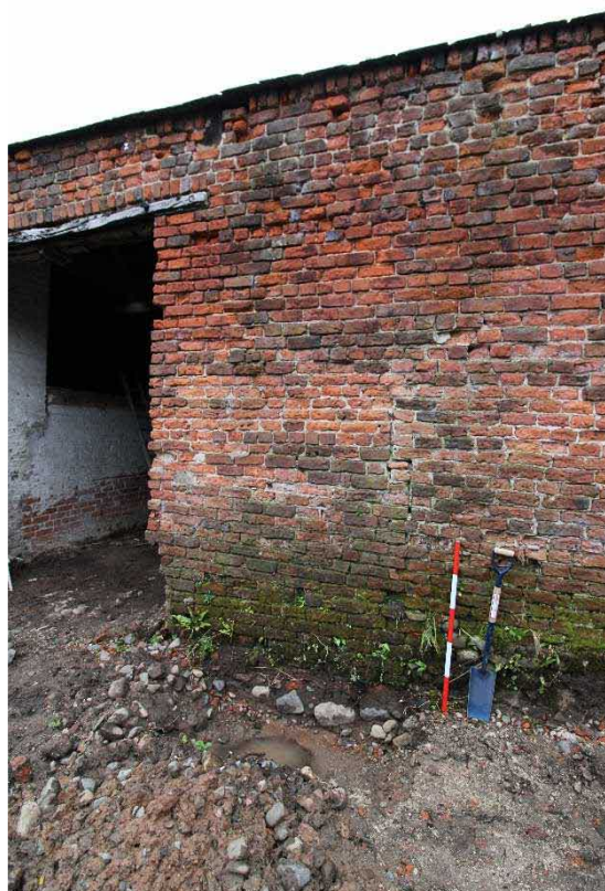
Plate 13: Construction break to south of cart entrance, with later brickwork above. Facing north-east, with 1m scale
