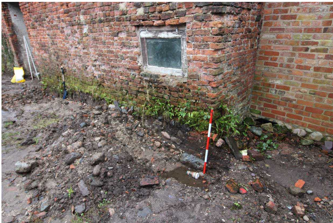
Plate 10: Inserted window at southern end of western elevation, facing north-east with 1m scale
