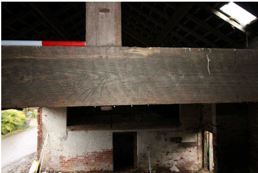
Plate 50: Baltic shipping marks on southern face of south truss, facing north with 0.2m scale
