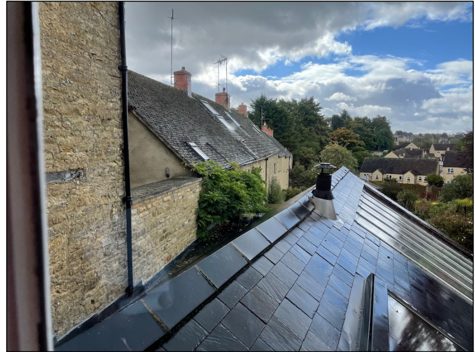
Figure 2: Roof of the kitchen (G5) extending above the modern extension and verandah of (G6 and G7).
