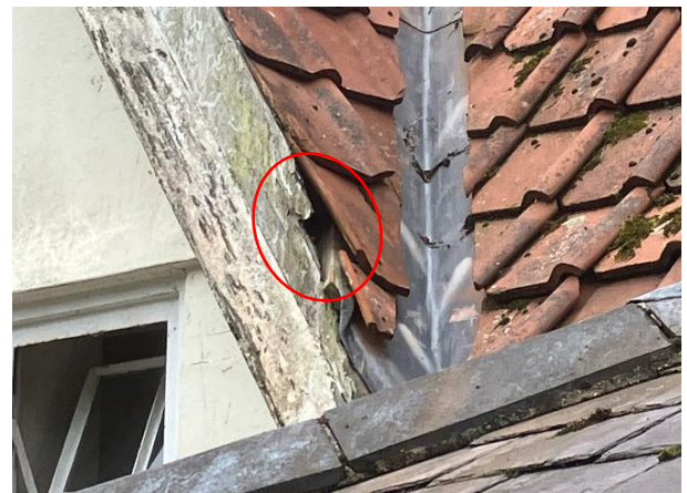
Photo 8: Gaps between tiles and rotten barge boards on northern façade of farmhouse
