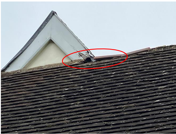
Photo 5: Potential bat access points around ridge and rotten soffits on eastern façade of farmhouse
