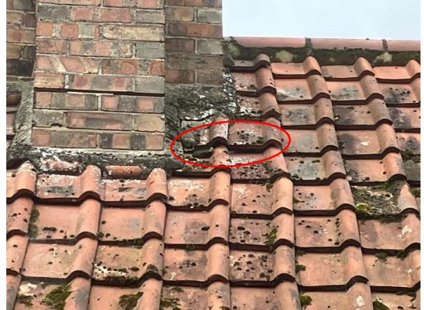
Photo 6: Gaps beneath tiles around chimney base on northern façade of farmhouse
