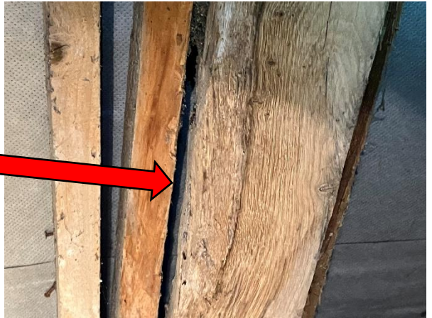
Photo 24: Likely location of roosting bats indicated by piling and pulling of roof membrane fibres
