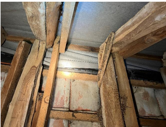
Photo 11: Ridge area of loft space, with breathable membrane running over ridge and c.200m down northern side of roof
