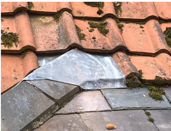
Photo 7: Gaps around tiles and lead flashing on northern façade of farmhouse
