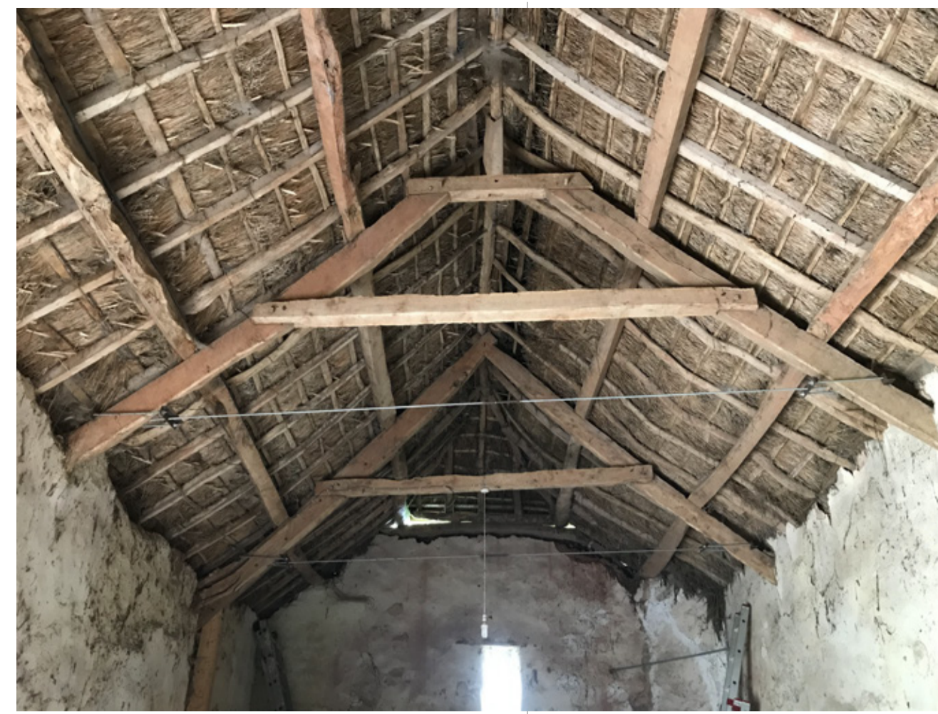
Existing exposed underside of thatched roof and existing plastered walls in need of repair
