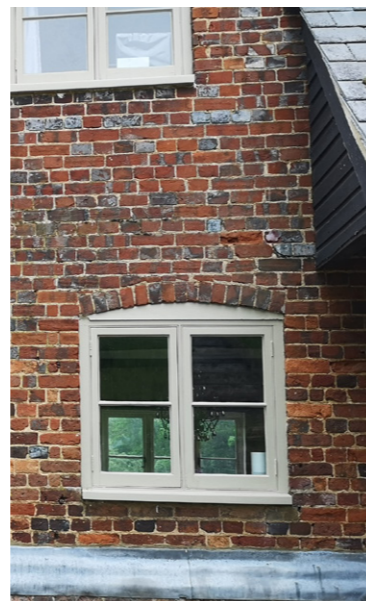
External windows and doors proposed in the existing dwelling, will be of a timber frame to match existing.
