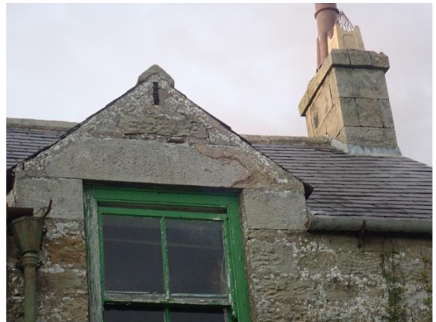
Occasional raised or missing slate
