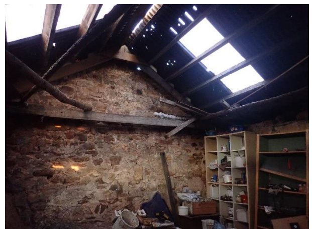
Interior of Outbuilding 1 with a very gappy roof
