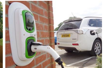
51 Electric vehicle charging points
