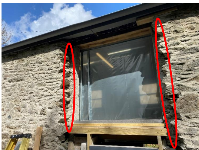
Photograph 9: crevices in stonework around windows
