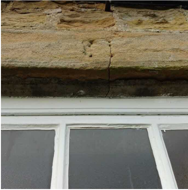
Figure 15. Cracked lintel to ground floor window east elevation of east wing
