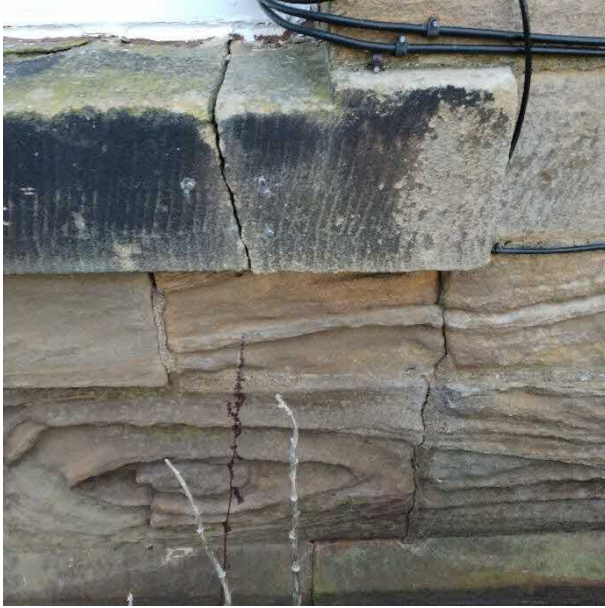
Figure 11. Typical cracking to stone window cills on south elevation
