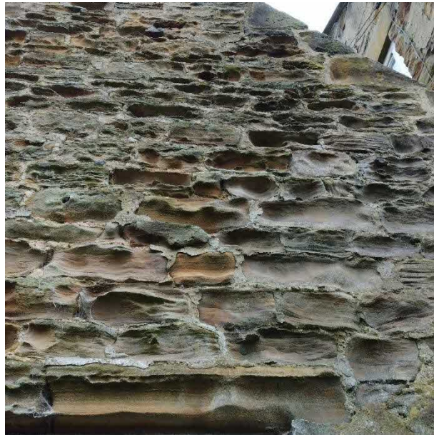
Figure 18. Example of stone erosion on north gable of east wing
