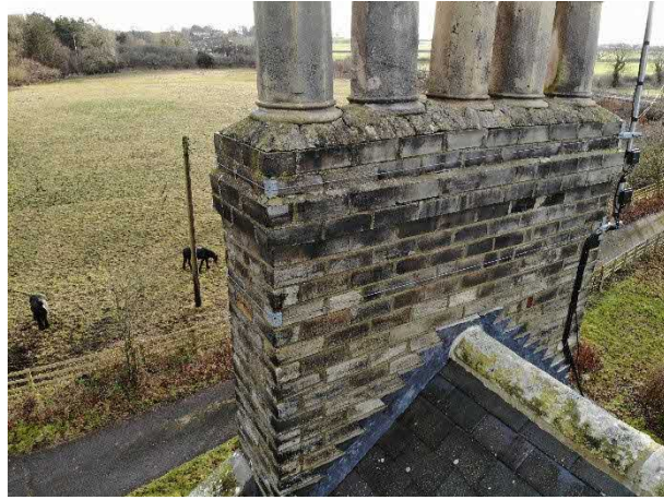
Figure 16. Cracking and movement to east chimney stack
