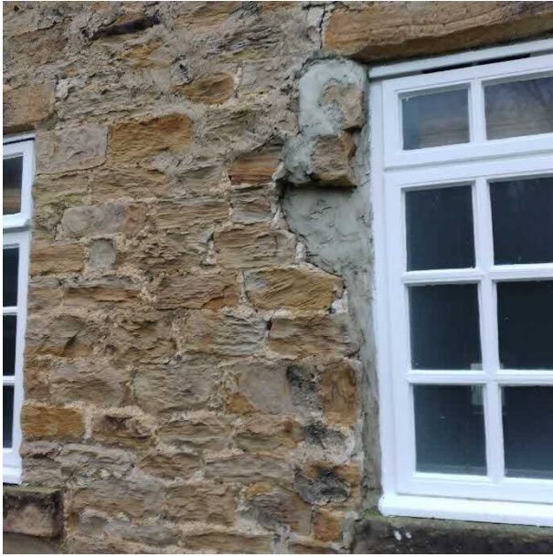
Figure 19. Poor condition stonework to west elevation of north wing.
