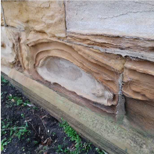
Figure 13. Example of stonework erosion on south elevation
