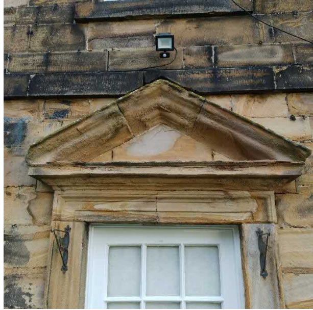
Figure 12. Cracking to lintel over central doorway beneath pediment
