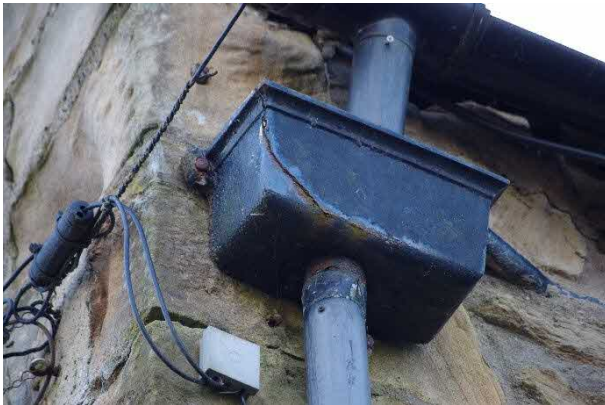
Figure 17. Broken hopper to north elevation
