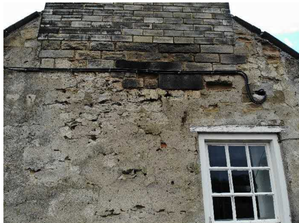
Figure 14. Deteriorating lime render to east gable
