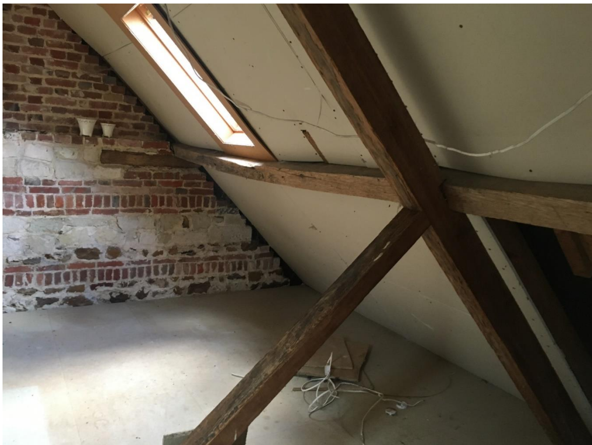
Figure 5: Timber embedded in the brick east end of the loft level and the purlin timber appears to be earlier than that used for the trusses
