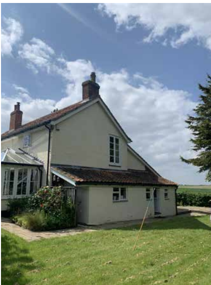
EXISTING EXTENSION TO EAST WITH GLAZED DOORS ABOVE; REAR ENTRANCE DOOR WITH STEP
