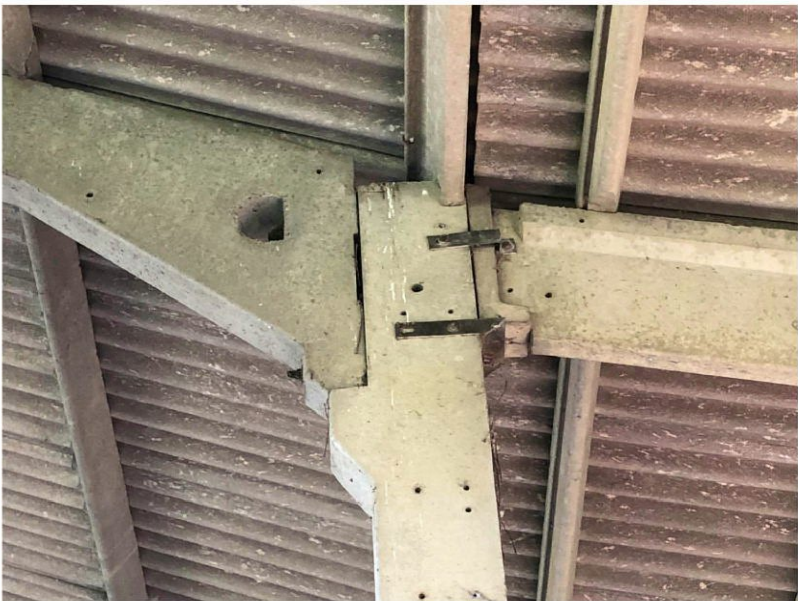
Detailed view on connection of post to portal rafter and lean-to rafter
