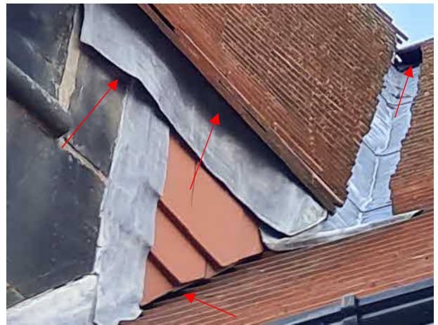
Figure 27: B2 - gaps under/between flashing, under hanging tiles and top of the valley of the dormer
