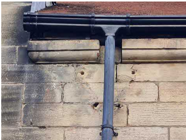
Figure 28: B2 - holes in the wall
