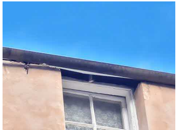
Figure 29: B3 - gaps above window frames
