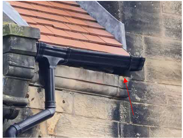
Figure 25: B2 - gaps under eaves
