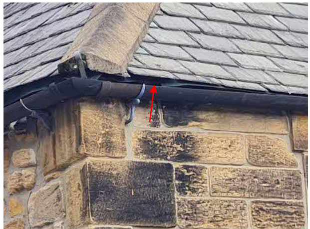
Figure 23: B1 - gaps under end slates
