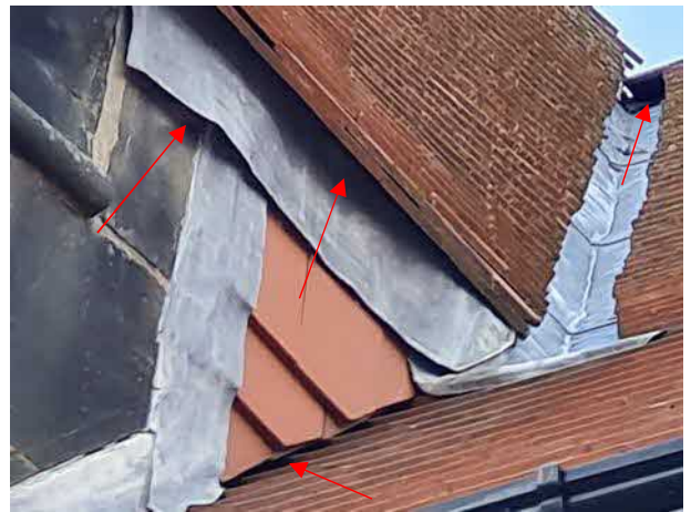
Figure 27: B2 - gaps under/between flashing, under hanging tiles and top of the valley of the dormer
