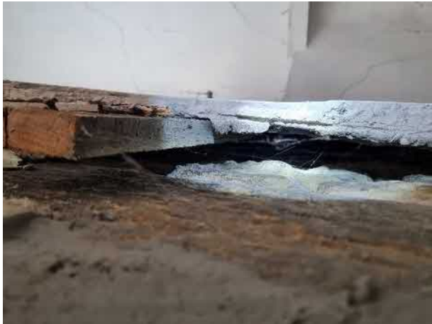
Figure 18: B2 - internal - wall cavity gap
