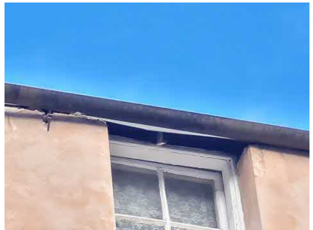
Figure 29: B3 - gaps above window frames
