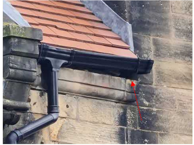
Figure 25: B2 - gaps under eaves
