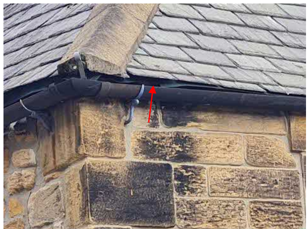
Figure 23: B1 - gaps under end slates
