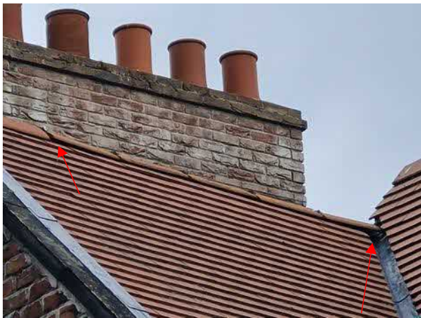
Figure 26: B2 - gaps under ridge tiles
