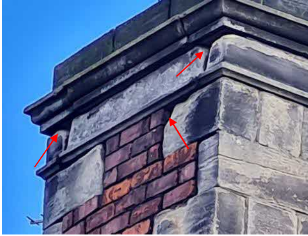
Figure 24: B1 - gaps in stones on chimney
