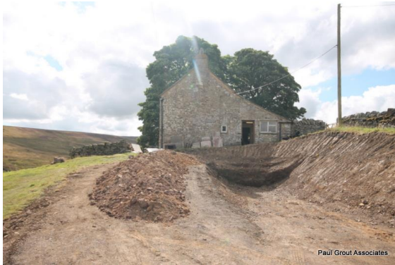
The garage is let into the sloping ground (earlier photo showing the excavation in progress) The roof only of the garage will be visible over the boundary wall to the track
