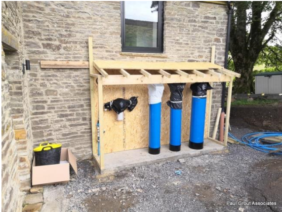
Photos of the unfinished enclosure for the water purification equipment
