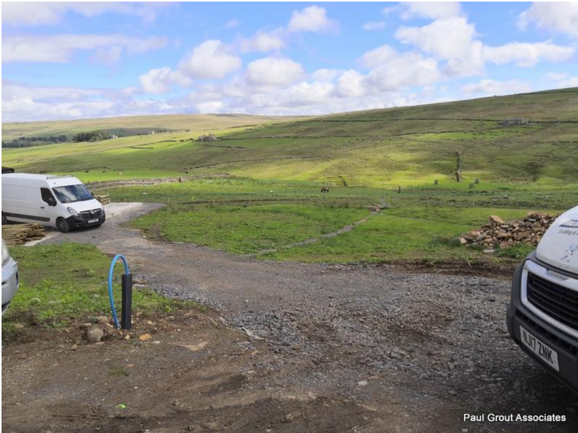
The new central drain (Drain 1) runs down the centre of this photo
