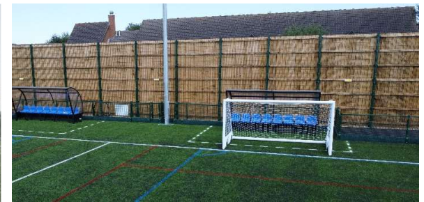
Example acoustic barrier
