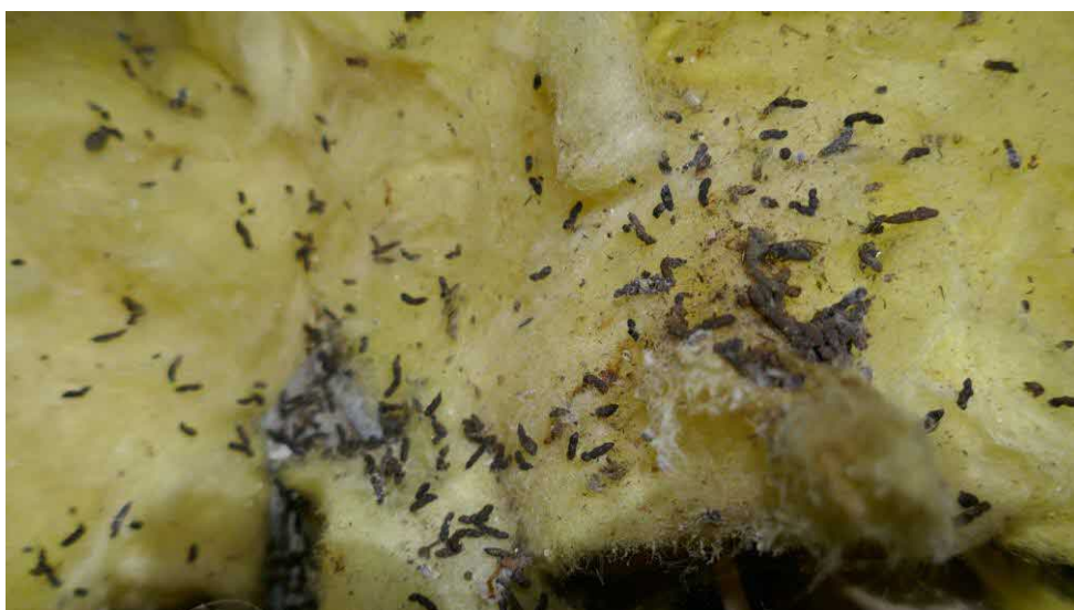
Figure 11. Bat droppings found in the roof void.
