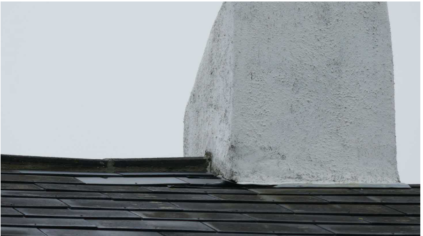
Figure 5. Gap beneath lead flashing around the base of the chimney.
