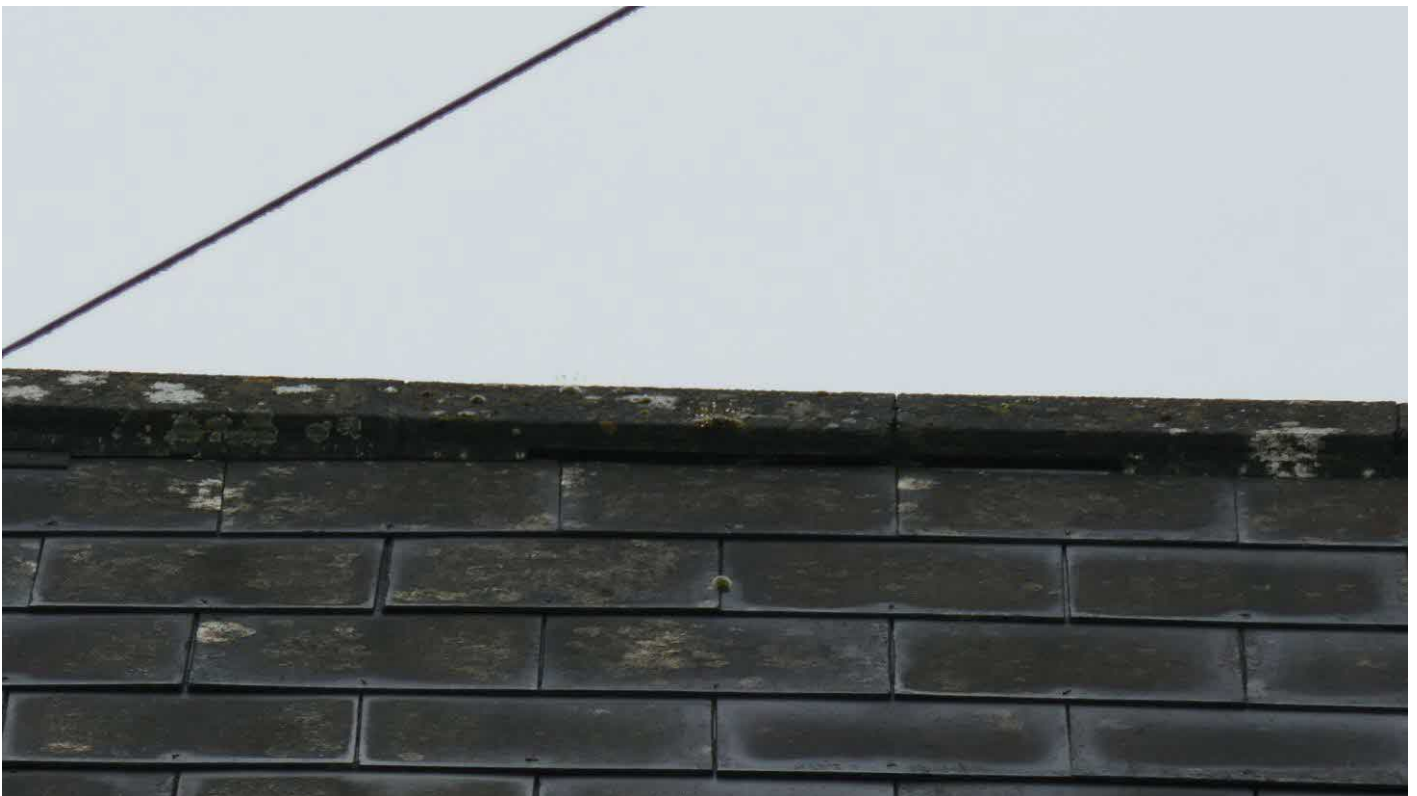
Figure 4. Gap beneath roof ridge.
