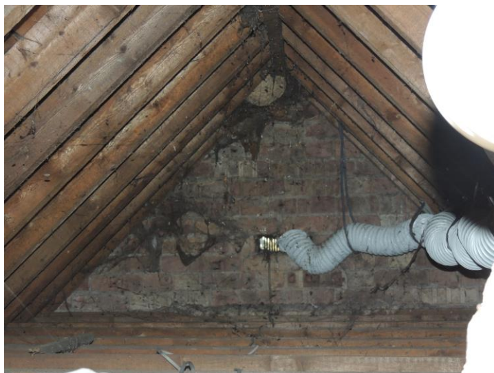
Photo 6: Note extent of cobwebs in loft
