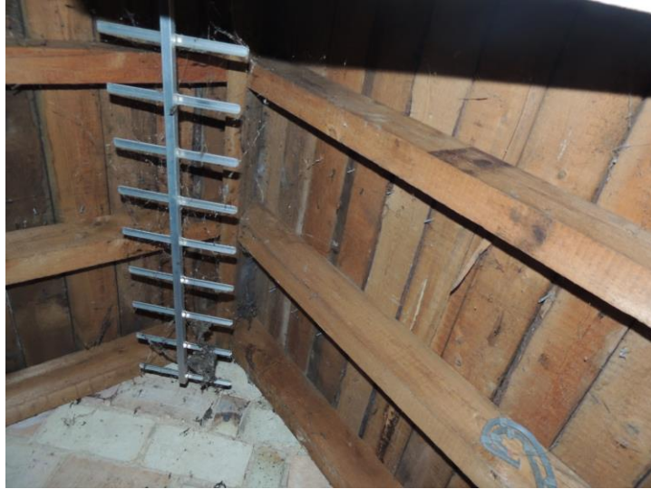
Photo 4: Note cobwebs on ridge of loft
