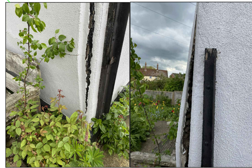
Main area of Delamination
