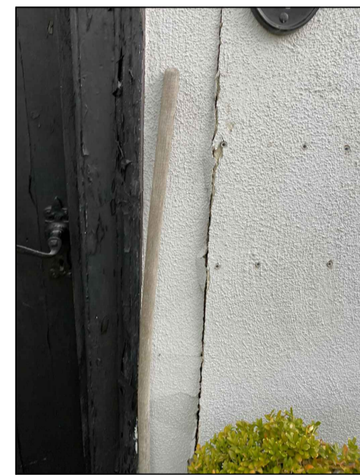
Beginning to Delaminate
