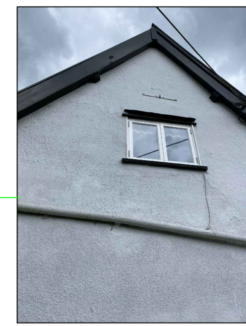
Painted Render to be replaced
