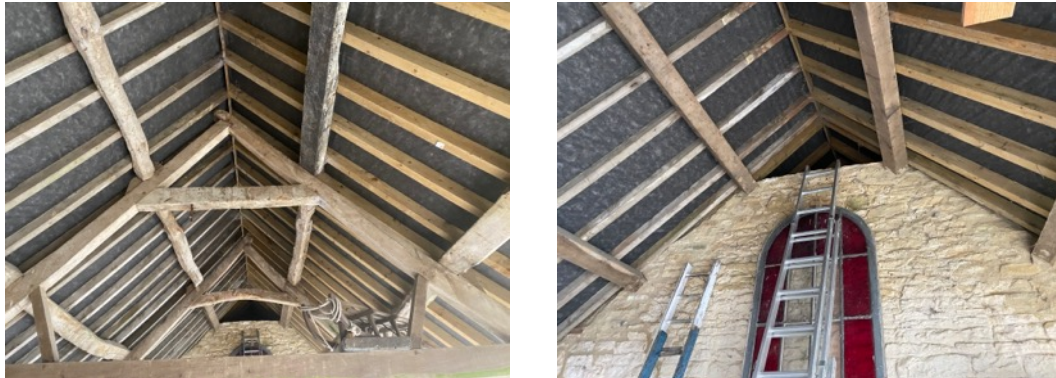
Figs. 7 & 8 Interior of barn and gap into roof void
